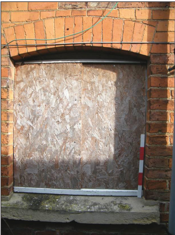
Plate 14 (Shot 24): Detail of window with stone sill and segmental arch on south elevation, looking north
