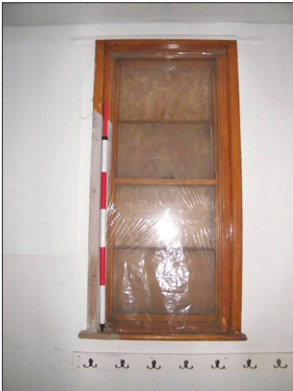
Plate 26 (Shot 38): Representative shot of sash window in south elevation of the old school room, looking south
