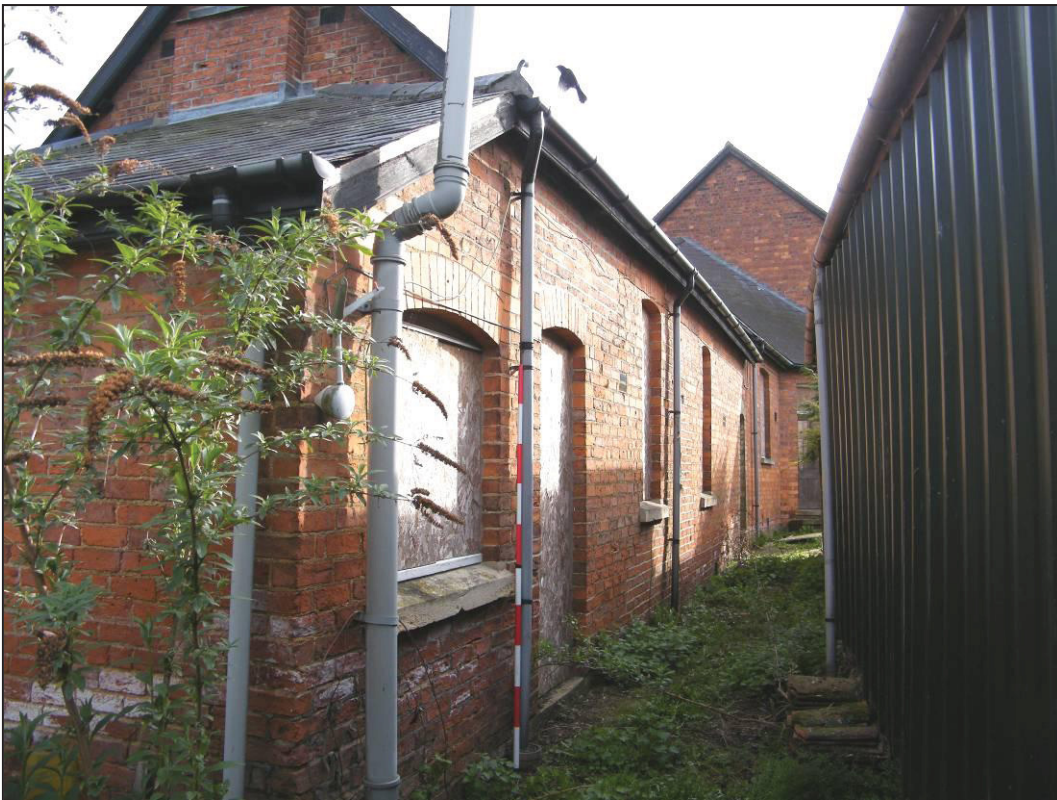
Plate 12 (Shot 22): General view along the south elevation of the earlier buildings west of the chapel, looking east-north-east
