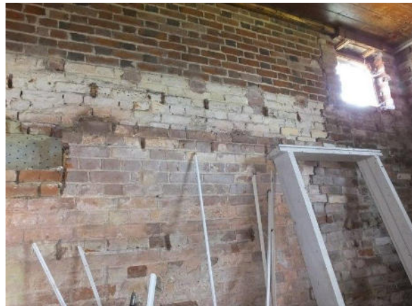
Side wall to the south shows timber plugs and lacing pieces to connect boarding for stable lining and floor for hay loft above.
