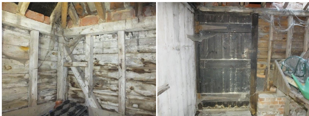
Tack room north-east corner detail. Eaves sealed. Original door to north wall of tack room.
