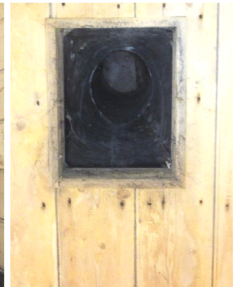
Ceiling vent end of tube.
