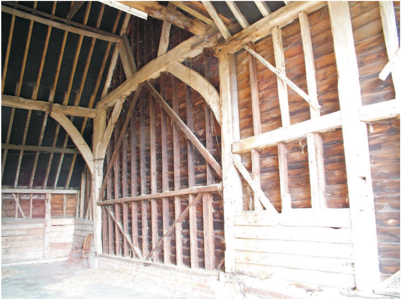
(287) South open truss showing late twentieth century infill when bays removed and structural elements possibly from the fifteenth century
