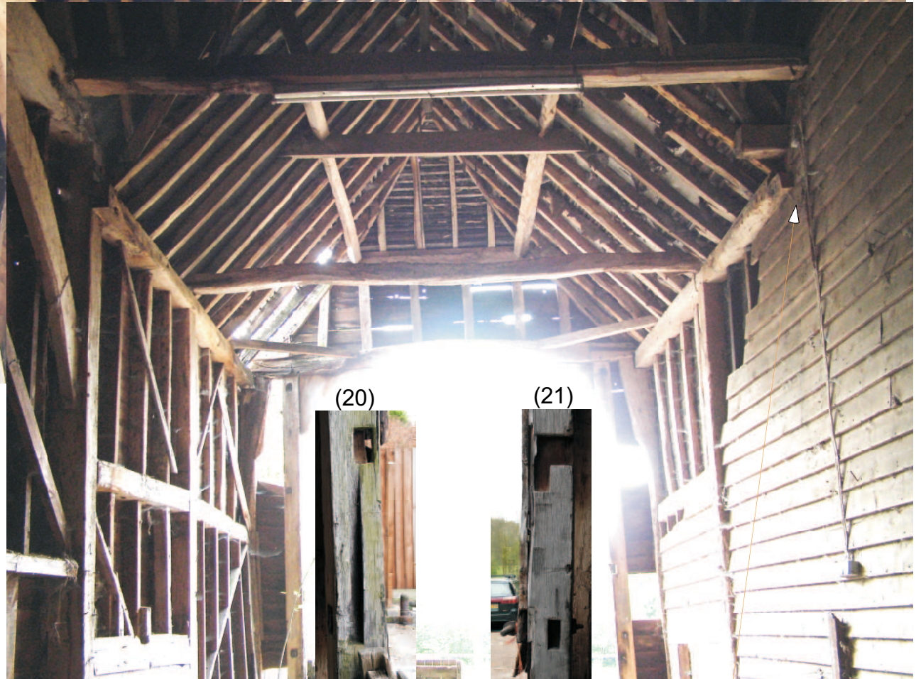
(295/296) South porch possibly seventeenth century origin. Inset shows mortises and cut-out for two types of retaining bar
