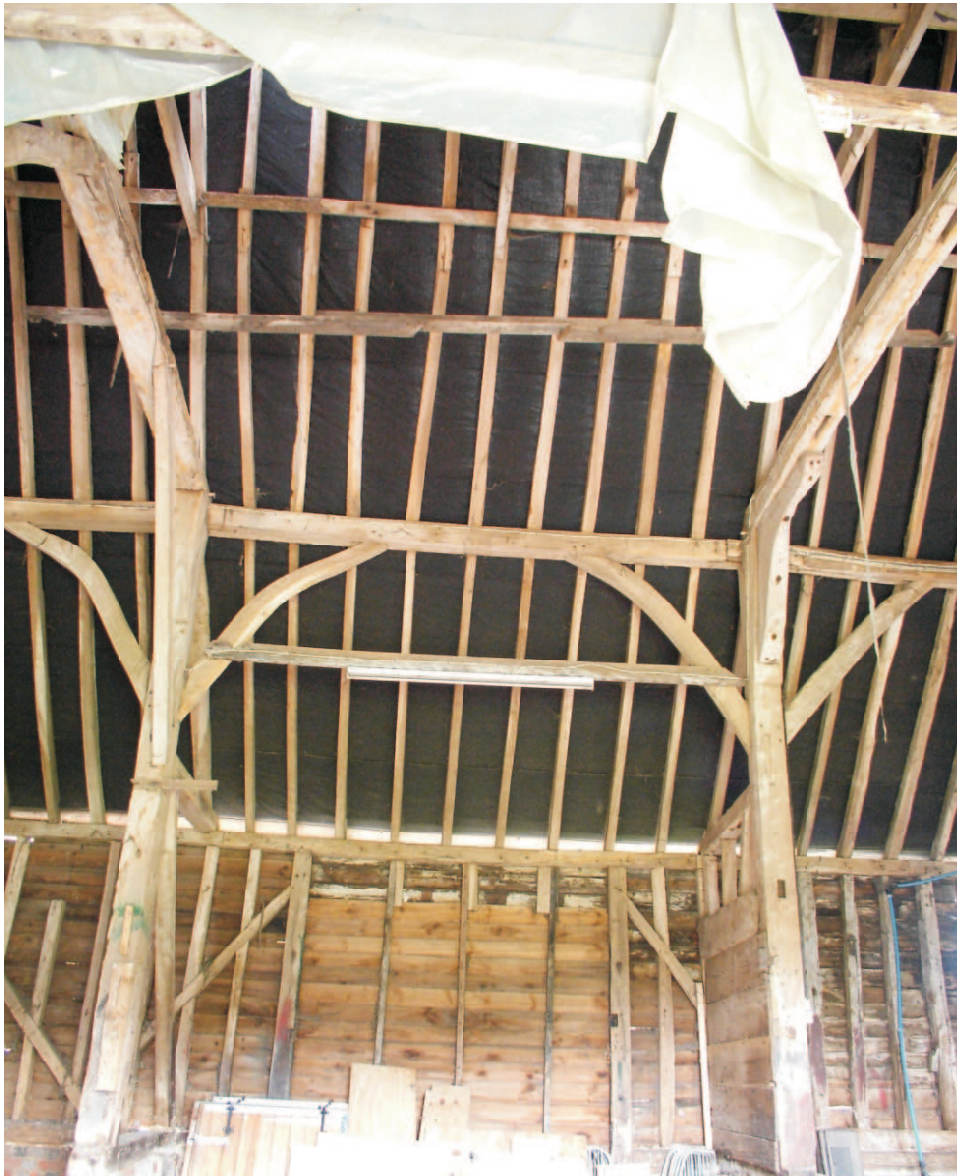
(255) Bay 5-6 east showing framing for opposing door to porch in eighteenth century build. Note that the primary bracing to the wall frame runs through to the next bay, The aisle wall frames do not relate to the main trusses but are built as independent units
