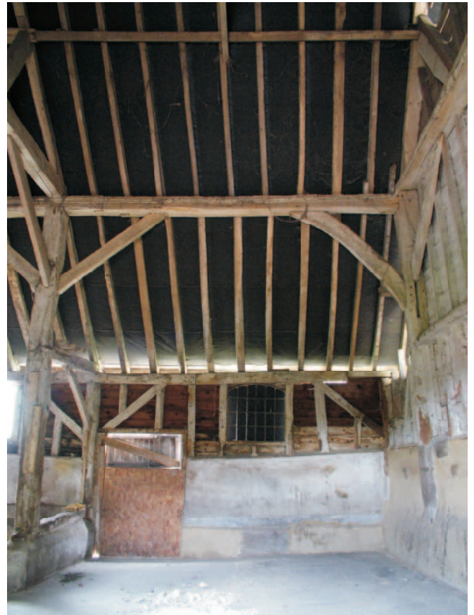
(238) Bay 2-3 to the east showing aisle wall framing for seventeenth century rebuild. note the arch bracing to the outer walls
