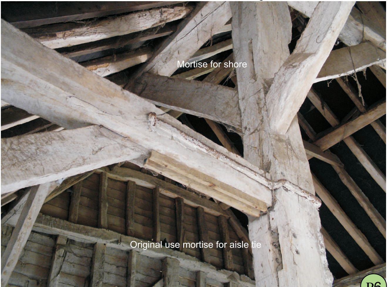
(248) View from aisle to post 3D showing in previous use had aisle shores.
