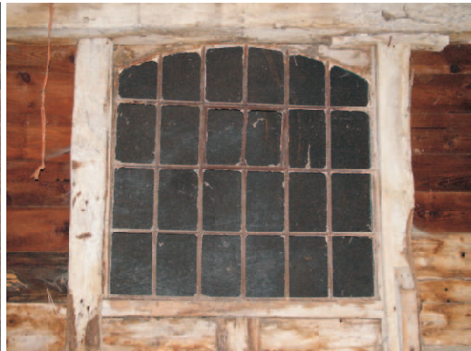
(145) One of two good cast iron windows circa. mid nineteenth century with opening vent.
