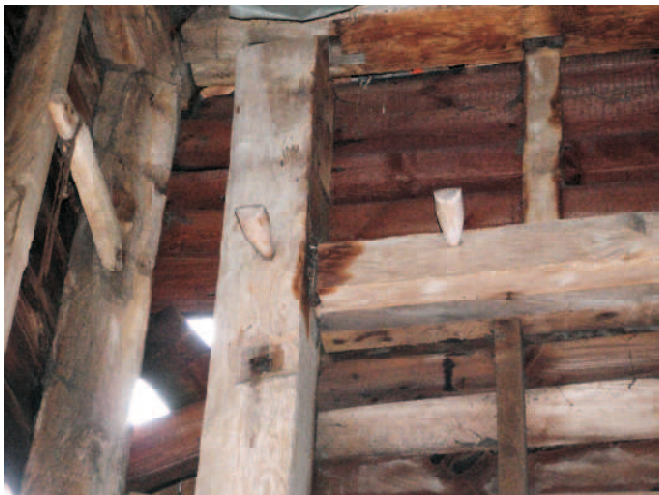
(177) Detail of side showing support pegs and end bar for pigeon boxes with late infill above.
