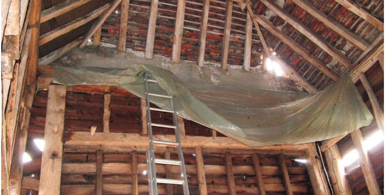
(178) Top of original door opening with line of pegs to support pigeon boxes.
