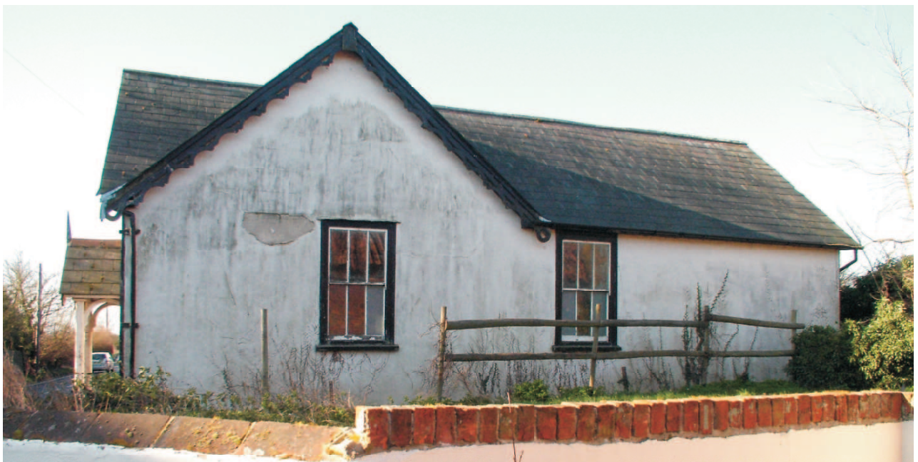
View from the north showing feature gable to the front with decorated and pierced bargeboards as the front. Two sash windows some still with frosted glass to the lower panes as on the front. Upper parts of wall lime rendered with ashlar marking. Lower levels re-coated with cement render. The roof covering is grey slate with a grey ridge tile. The porch has red ridge tiles.
