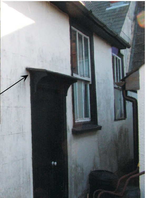
View along west side to junction with adjoining cottage. Note ashlar stone finish to plaster.
