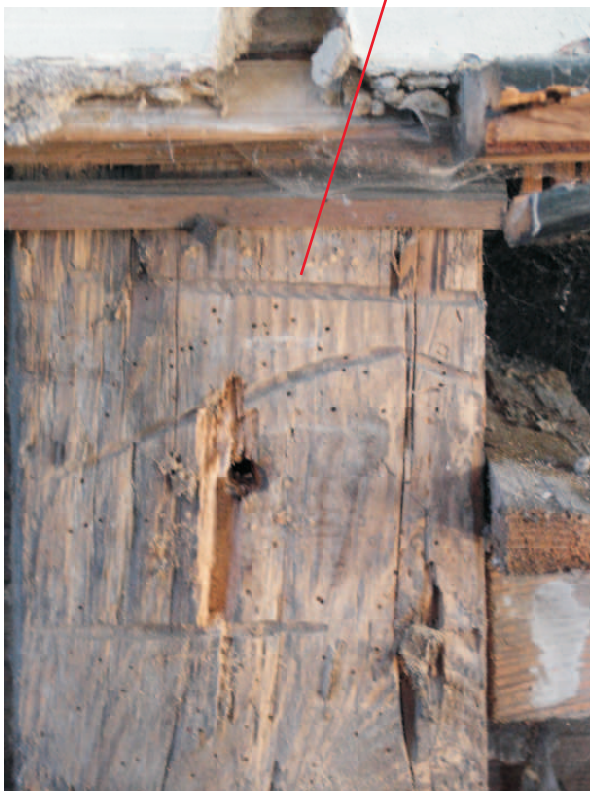
Example of bracking marks seen on the larger sections of timber
