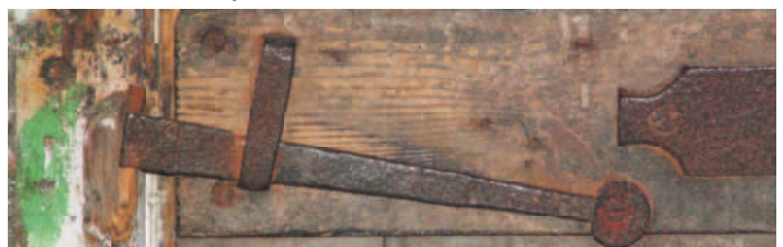
Lower latch still in place
