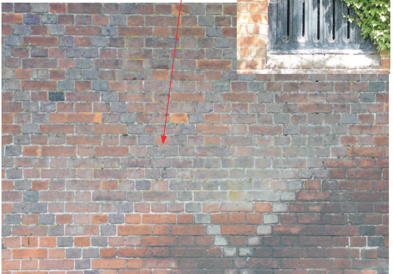
West elevation of building (facing the main road) with diamond diaper design in brickwork using flared headers. A large cast iron vent to the stable end of the building. The rear lean-to with an original doorway and the brick bond changing to Monk bond.
