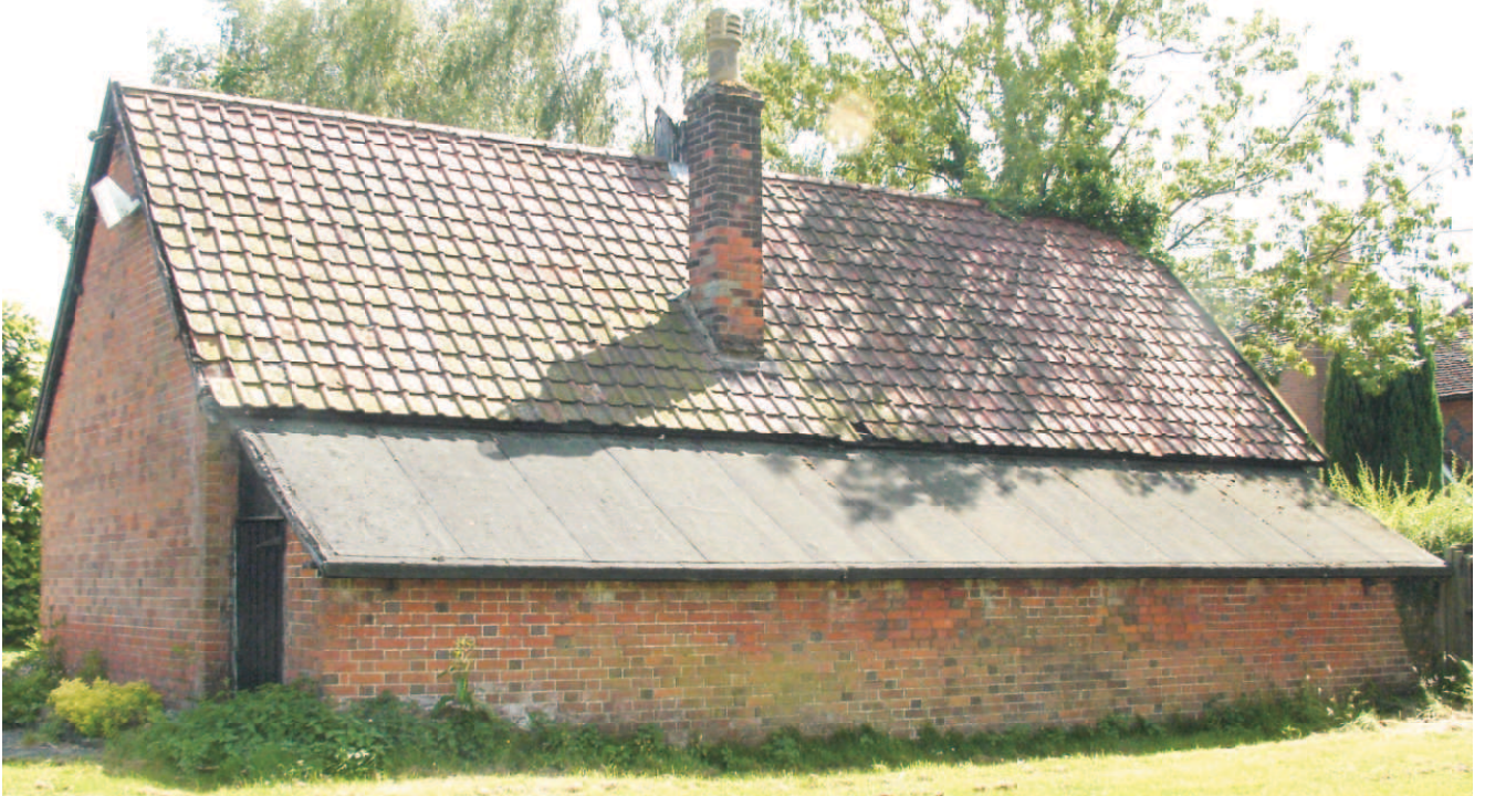
Rear elevation, with east end below. Flemish bond brickwork to east & Monk bond to north
