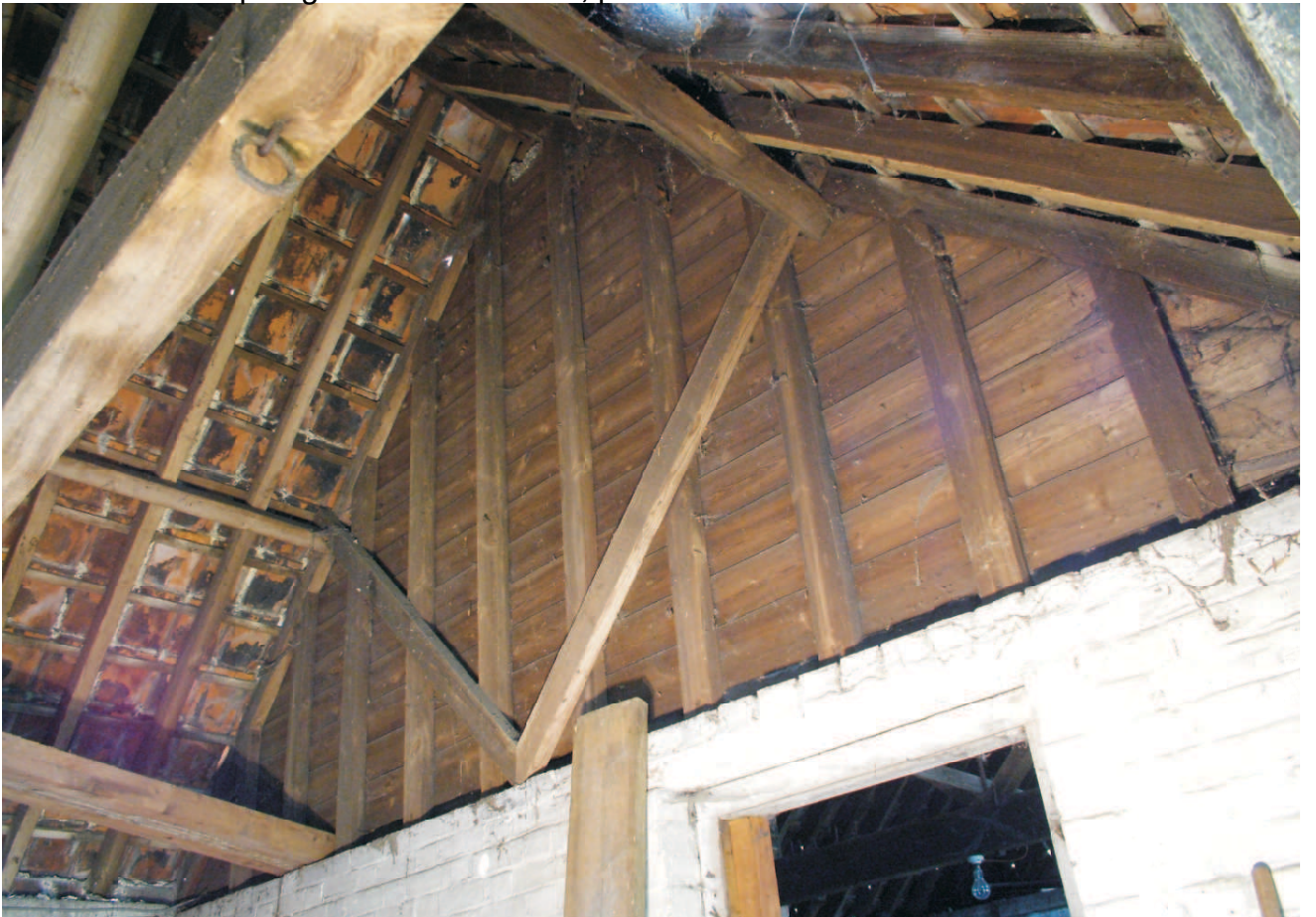
West end view up to intermediate wall and board infill above wallplate. Struts from purlin to wallplate. Note iron ring hanging from tiebeam
