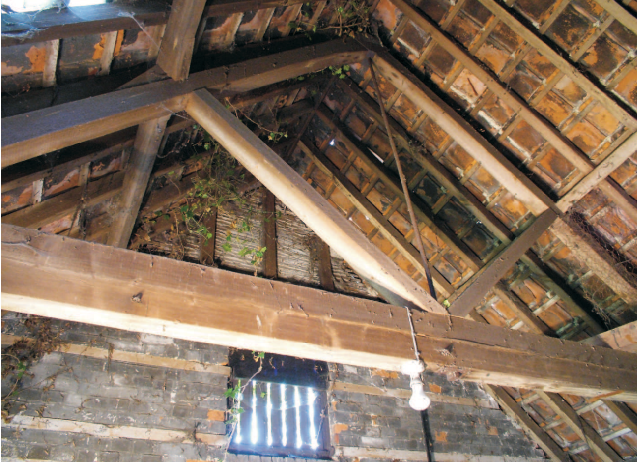
West end view up to gable with cast vent, plaster infill & main truss across centre of area.
