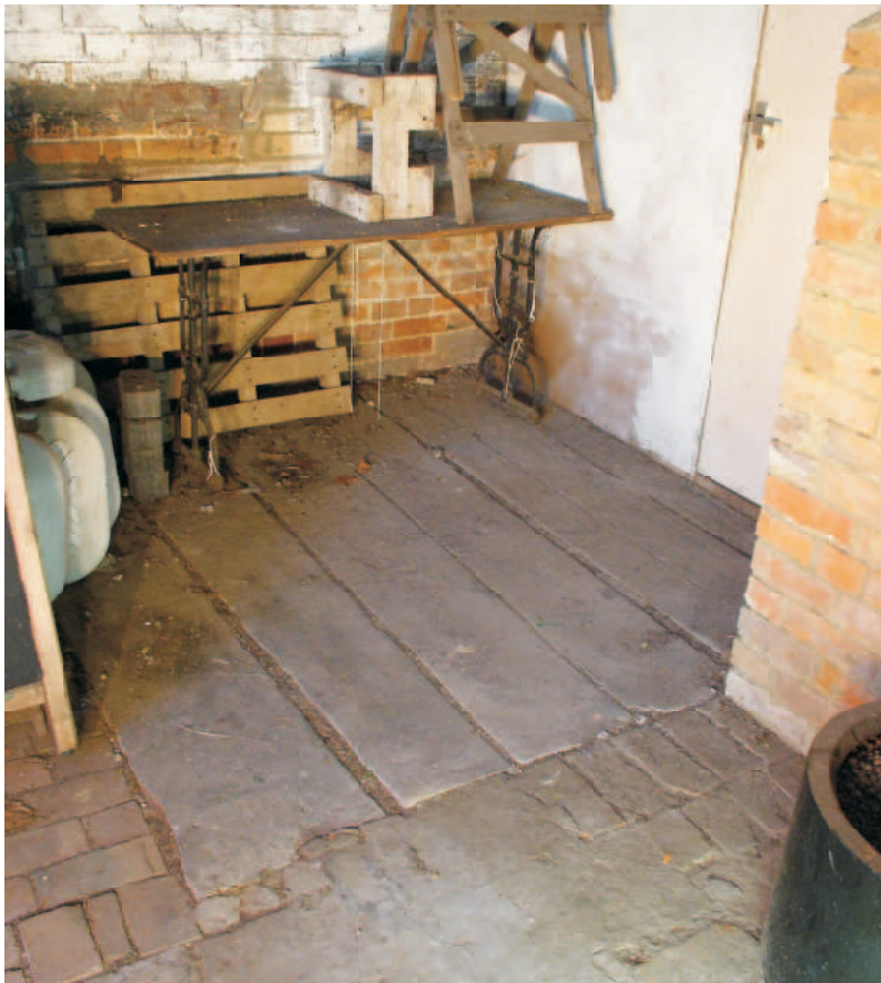
Remaining boarded area with last board broken as it crosses hearth area
