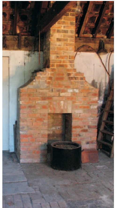
Rebuilt hearth area with modern partition now closing off open wall to lean-to
