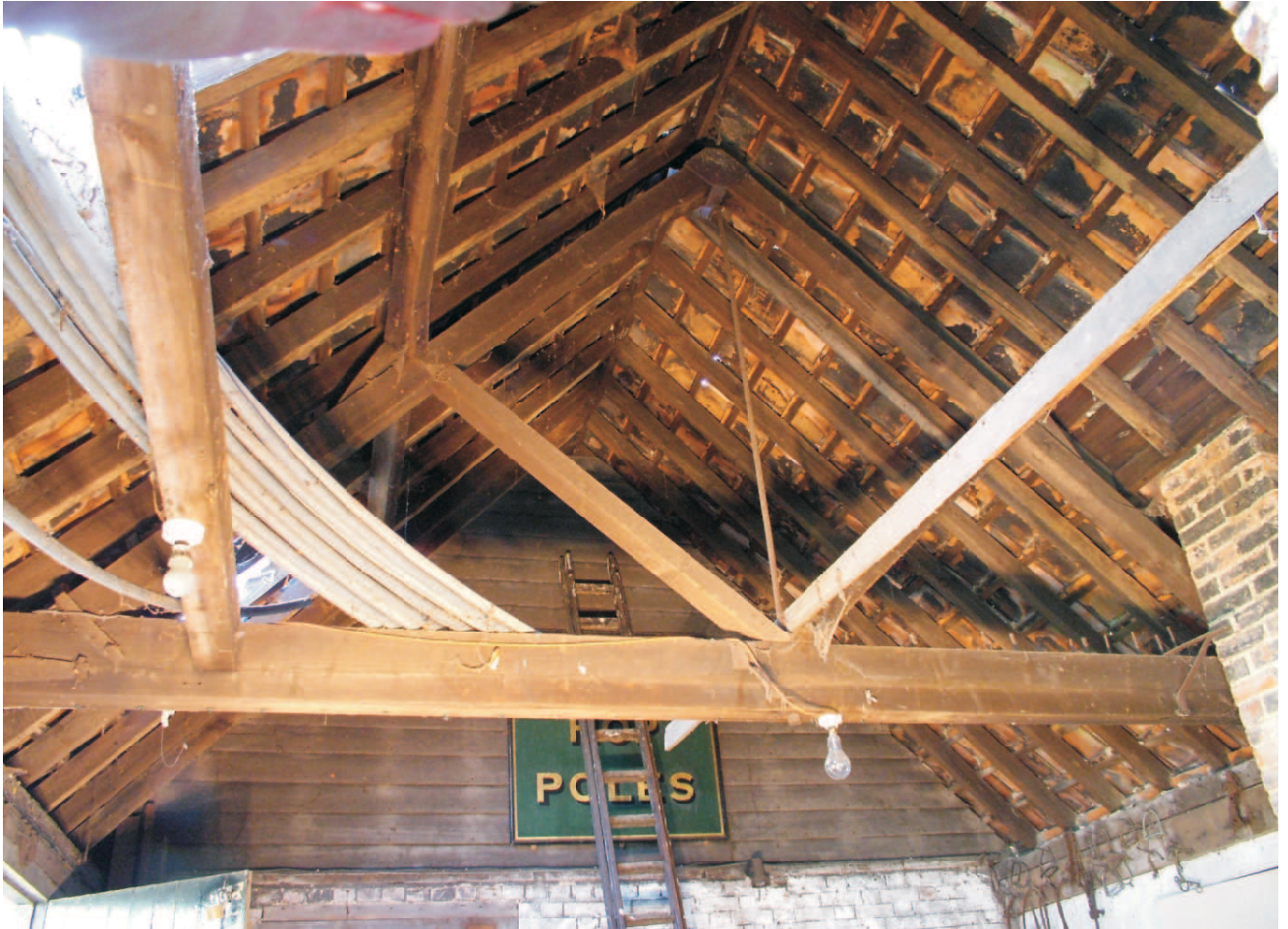
Roof to central area with main truss, axial beam to east and boarded infill & sign to west
