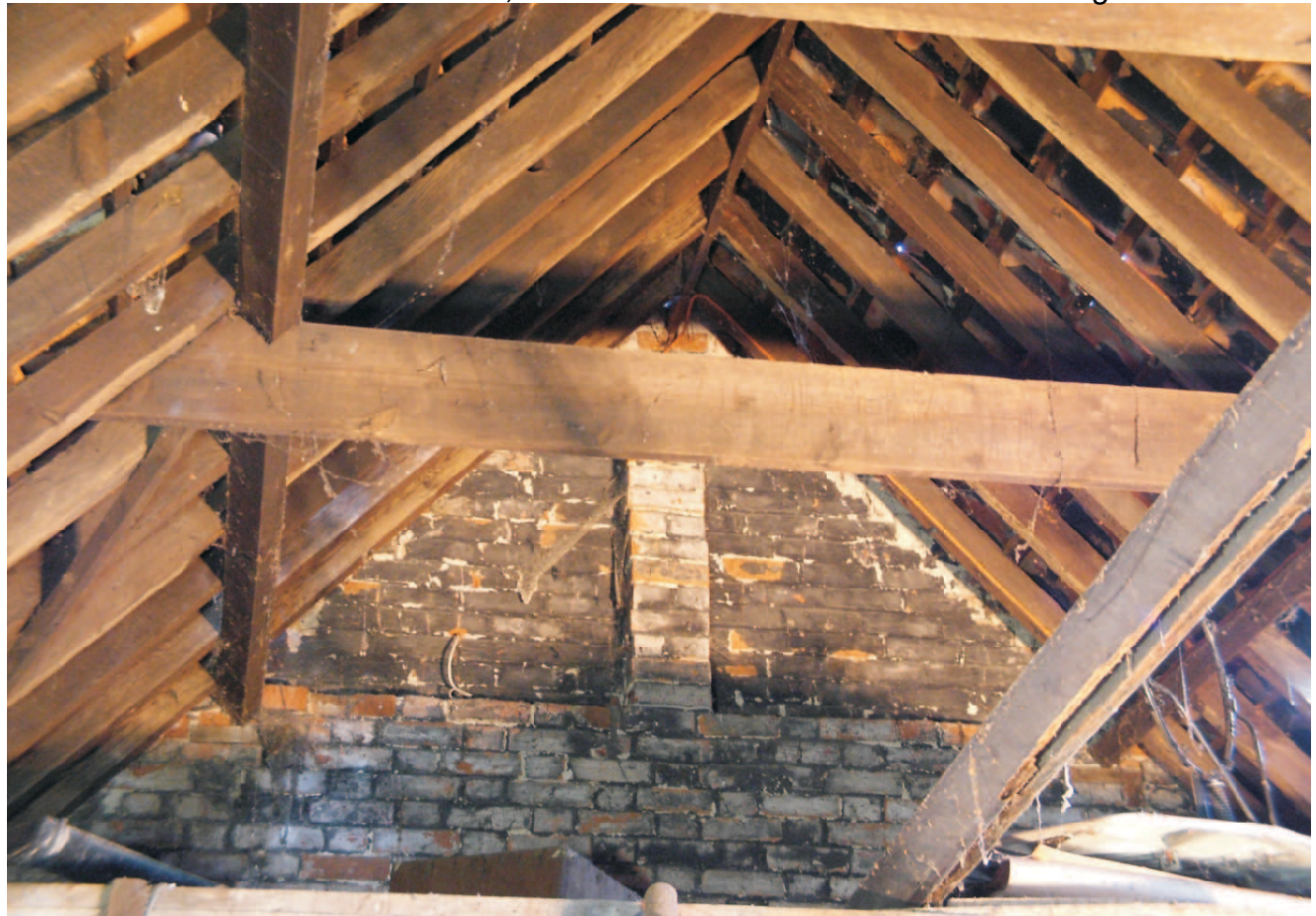
Roof from central area to over eastern area with collar roof and lower rafter brace, top end gable half brick with pillar. This area may have been for storage.
