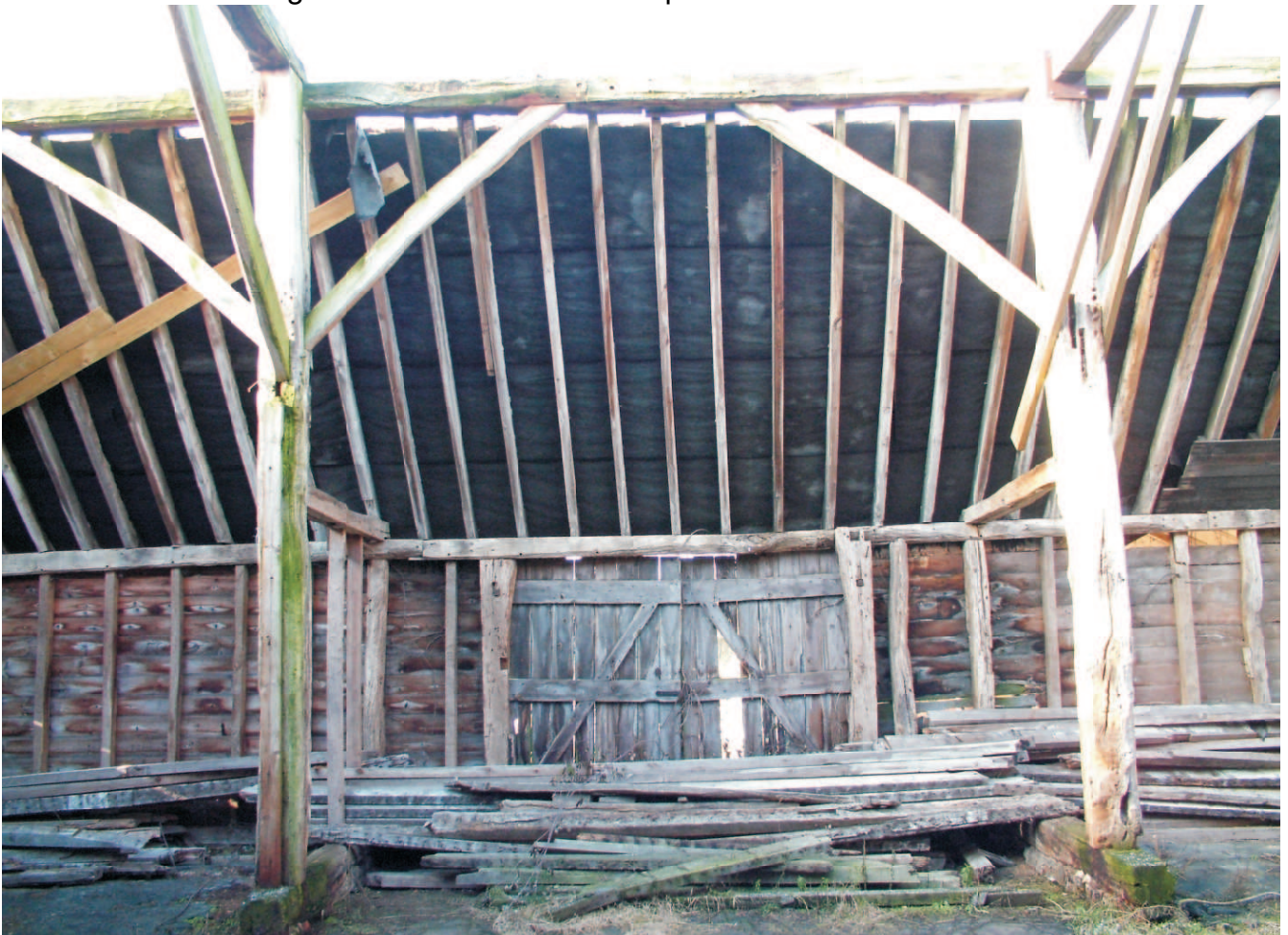
Barn, A. View to west aisle showing extended width rear nineteenth century doors opposite each of the midstreys. Aisle wall to right original, to left rebuilt in nineteenth century.
