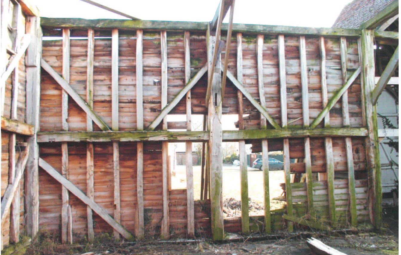
Barn, A. View of two northern bays on the east wall. Shows the typical primary braced frame structure found through the barn. Note reused toplate as midrail.
