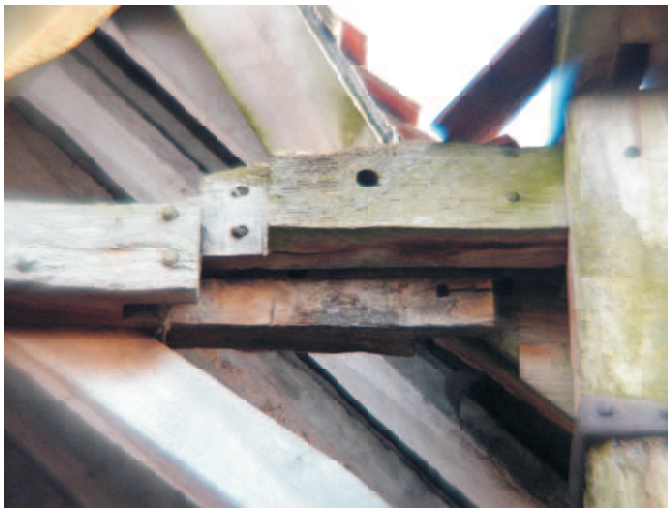
Barn A. Typical face halve and bridled scarf joint with double pegging and large key peg found in topplates and arcade plates.
