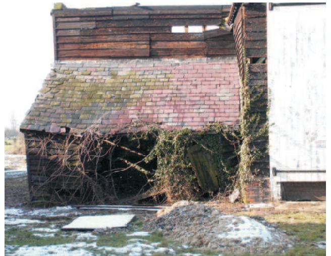
Barn A. Outshot to south-east corner of the barn, nineteenth century with slate roof. It has doorways to east, south and into barn.
