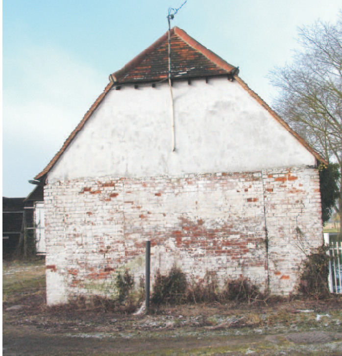
Building B. View on east wall. shows two parallel breaks for original wide carriage entrance. Infilled vents either side.
