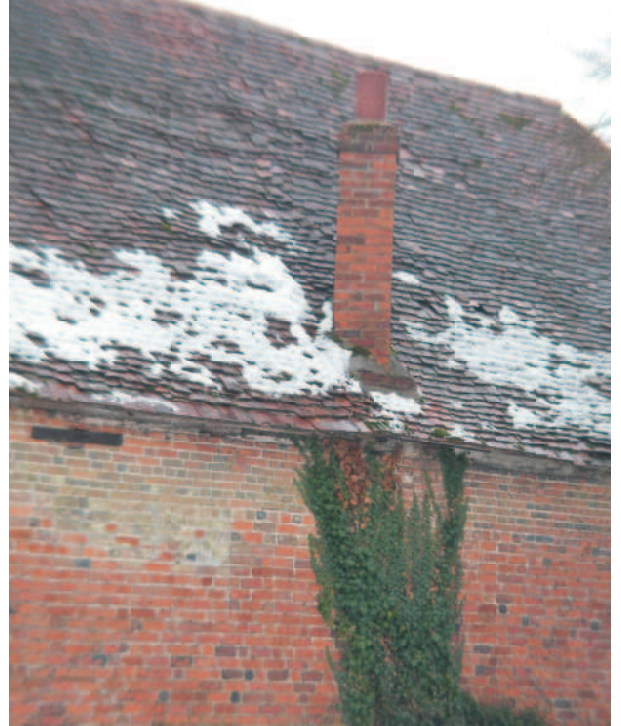
Building B. North wall showing diamond set Tack Room stack and iron tie through building.
