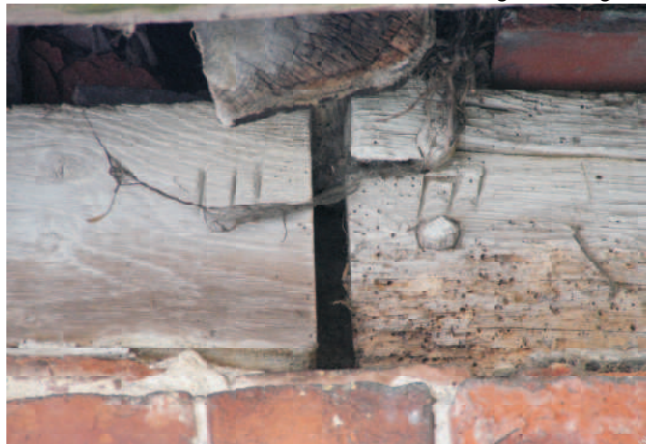
Detail of topplate bridled scarf visible in north wall near stack. Carpenters chiselled marks III.
