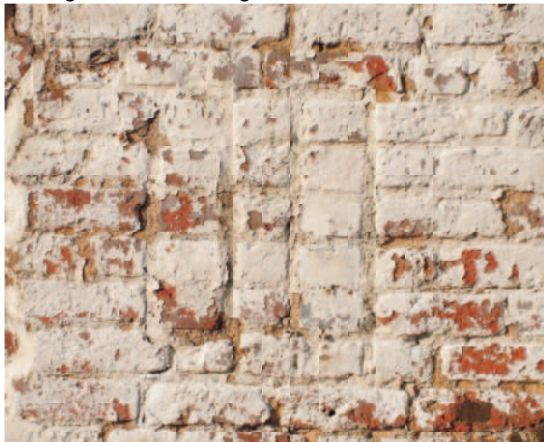
Building B. Detail showing one of infilled brick vents in east wall.
