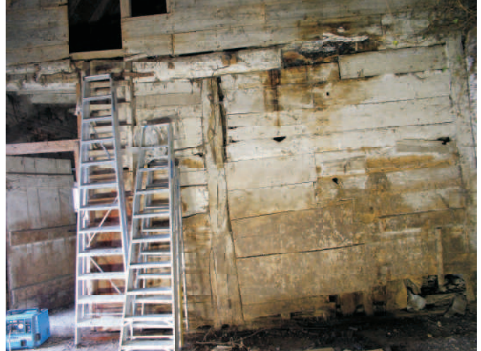
Lower area of division wall with wide board infill and doorway to Nag stable.
