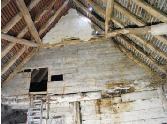
Building B. West division to Nag Stable and Hay loft entrance above. board & plaster infill.
