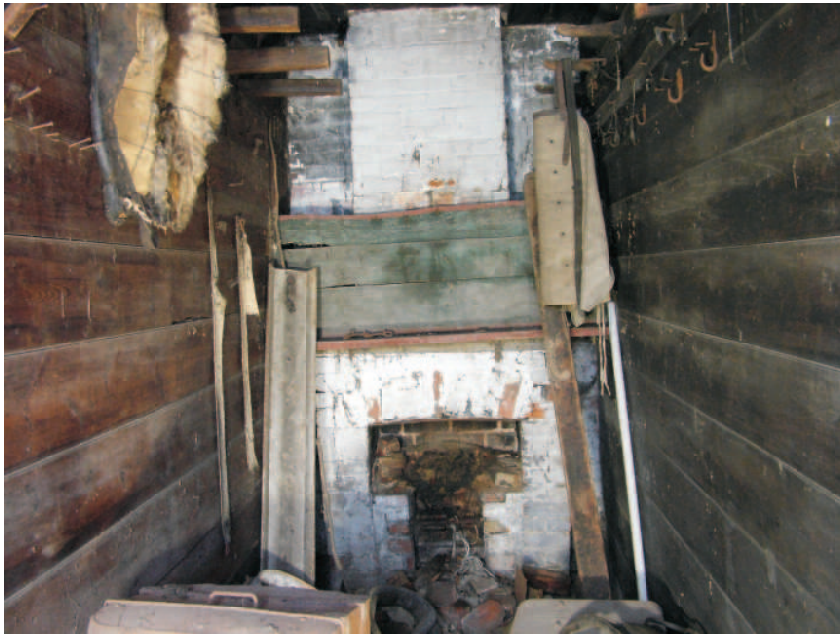
Building B. Tack Room. View to north and brick fireplace. The side walls are fully boarded with good wide softwood boards.
