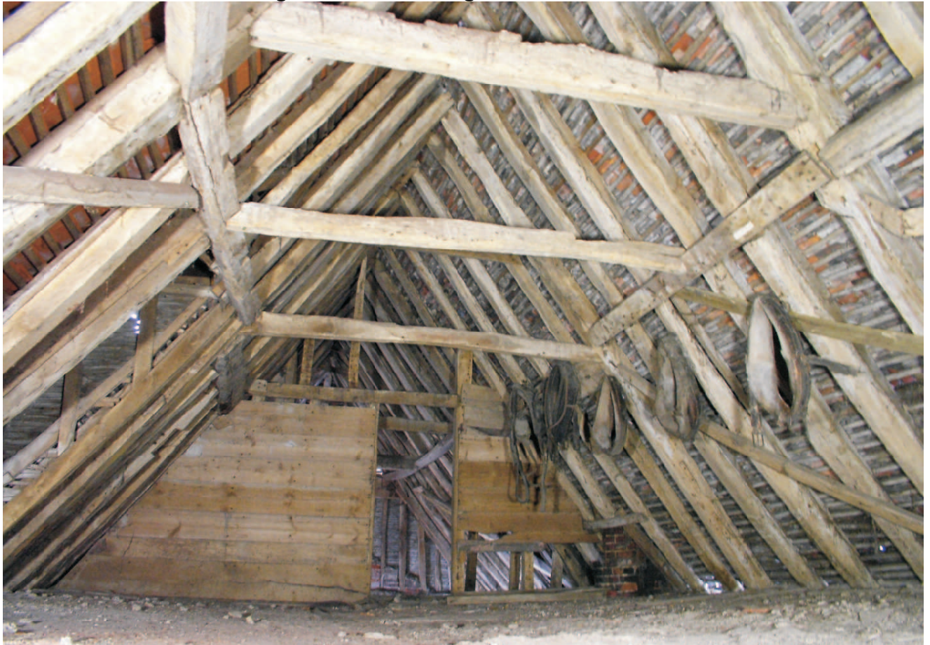
Building B. Hay Loft with view to west and access to gallery above Carthorse stable. Framed side purlin in area where stack goes through roof.
