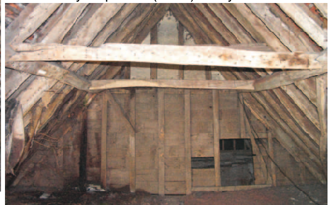
View towards carriage shed vertical ladder access with framed boarded infill and plaster above collars.
