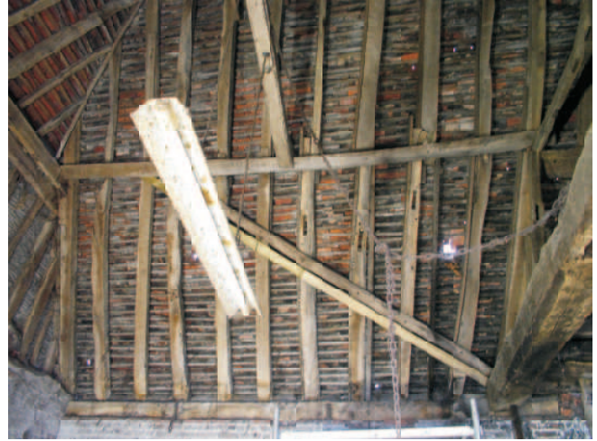
View to rear, north, roof shows reused timber & poor structural features.
