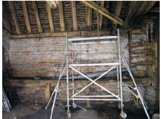
Rear wall, north, with feed trough and rings for five horses. Shadows show where hay rack was fitted.
