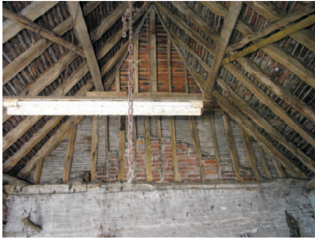
Building B. End wall of Carthorse stable, shows brick gable of adjoining build & a mixed infill around it.
