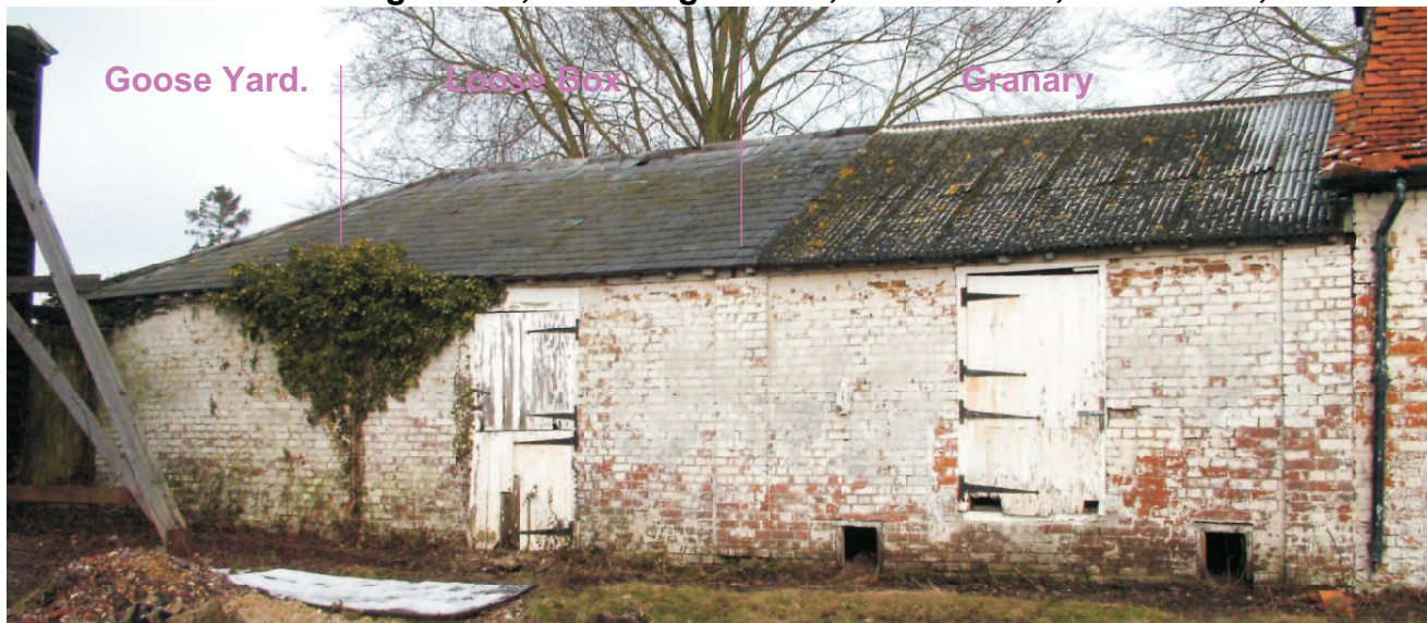
Building Range B. West building. The three pillars designate the room divisions. Raised floor granary to east.
