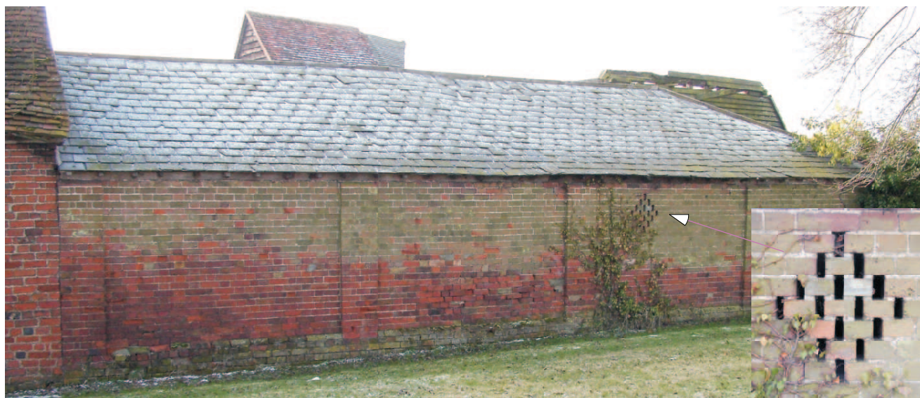
North wall with four pillars , no room designation. Plinth in English bond with shouldered plinth bricks between the pillars. The detail shows the brick vent to the loose box. Slate roof, all structure nineteenth century.
