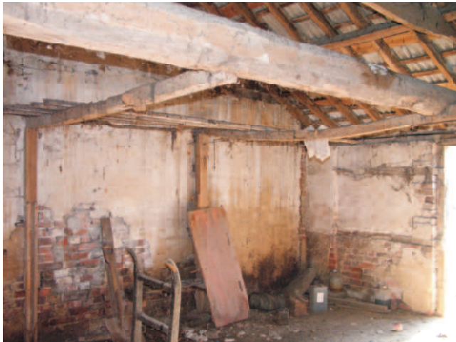
View to front south east corner showing broken brick joint suggesting Carthorse stable was originally longer. The large detail shows the same area on the outside with broken brick forming the end of the stable wall.
