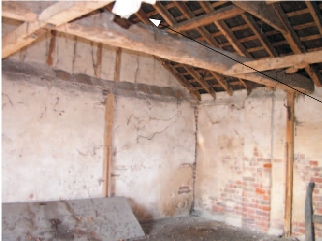
View to north west corner showing plastered walls and infilled eaves against rodent entry. Vertical timbers to walls with fillets for division boards.
