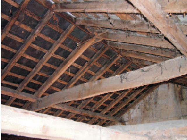
Building B, Granary. Detail of side purlin roof with collars to principle trusses and consistent size rafters. The raised ridge board was for a lead formed ridge.
