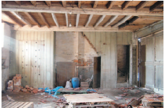
West inserted wall with fireplace in centre, cupboard to south and stairway to upper floor living room to north.
