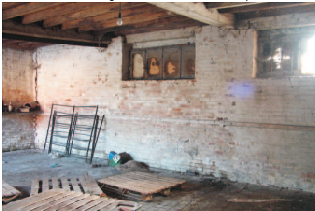
Rear, south, wall with modified windows. Shadow for division wall below beam. Later dado rail. Brick floor.
