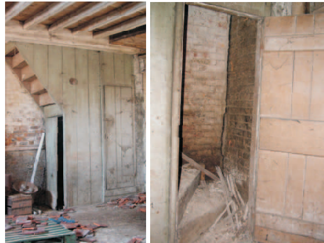
Boxed stairway detail with door closed and open, most likely later eighteenth century.
