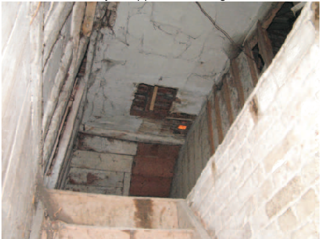
View up stairway to landing above with hole in ceiling from where chimney stack has been removed.
