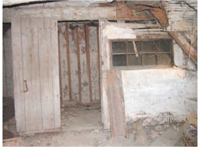
View from living room through door to landing. Note window for borrowed light to stairway.
