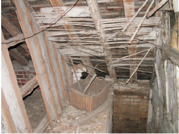
Building C. View down stairway from landing. Basket is on top of inserted division wall.
