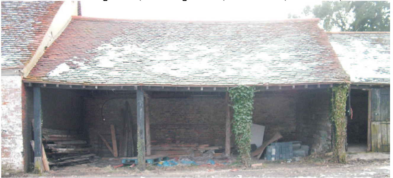
Buildings C. Cartlodge linking the buildings and against the garden wall. Plain tile covered modern roof.
