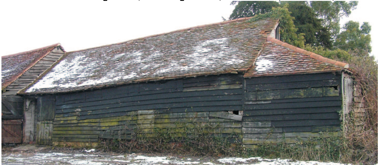
Building C west building. The Cowhouse timber framed & weatherboarded with later lean-to and plain tile roof.
