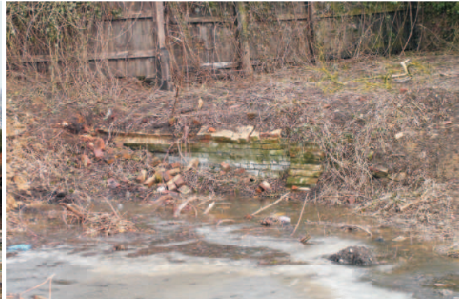
Looking across the north boundary pond and towards the area to the west of the Goose yard building. The failing revetment to the pond may have been the end of a bricked area beside the pond.
