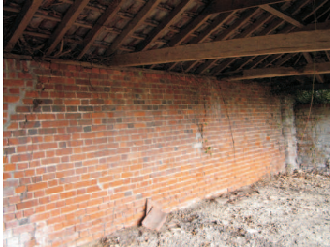
Rear wall of west shed with good brickwork. End wall from earlier building, earlier brick.
