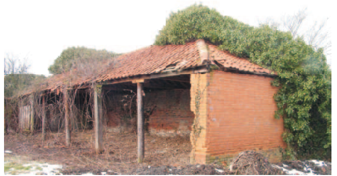
Eastern shelter shed with rebuilt east return wall. roof is covered with single Roman clay tiles.
