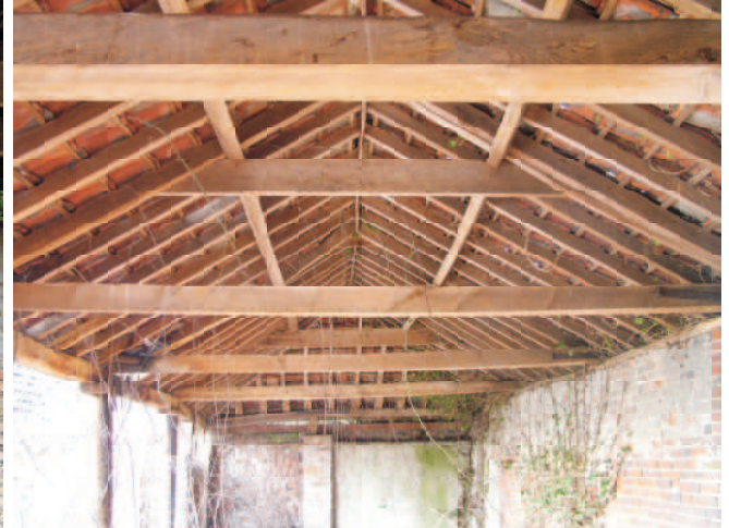
Typical roof structure in shelter sheds, nailed collars, constant sections and ridge board, this is the east shed.
