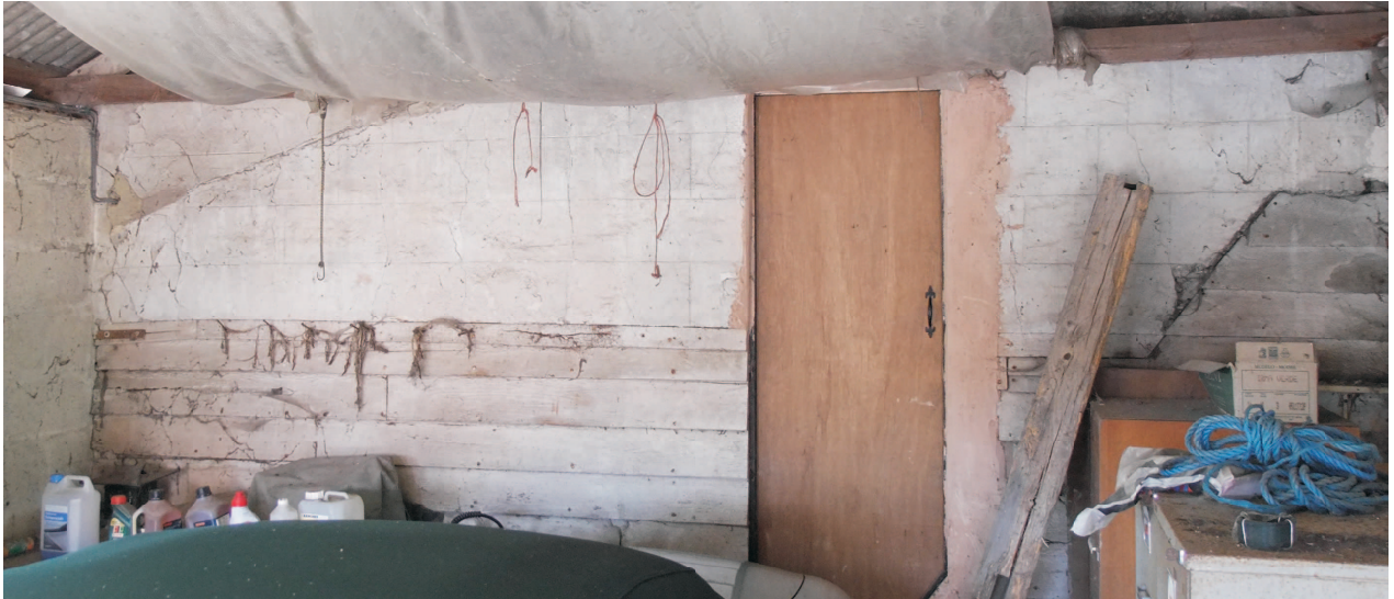
Granary east end with ashlar plaster to house. Late door insertion from modern garage. Note structural brace line in plaster and at bottom of door. Weatherboarding to left of door appears to be original.
