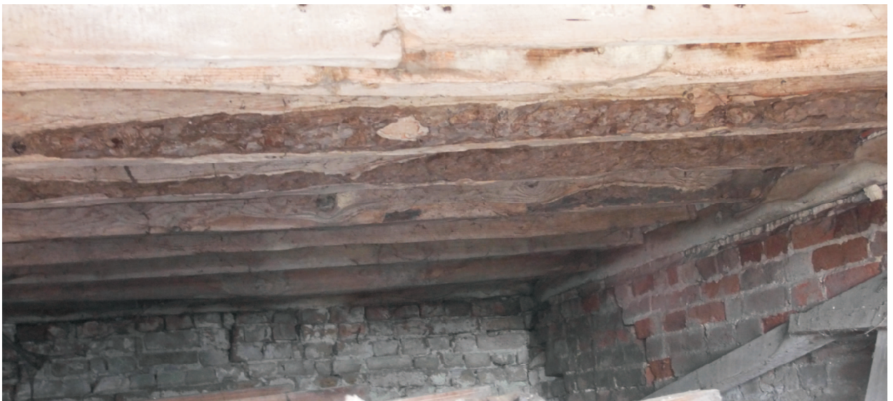
Granary under view showing north retaining wall against slope and intermediate pier wall. Note the amount of bark surviving on floor joists showing how maximum possible section was being produced from limited size trees.
