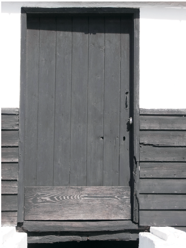
Granary entrance door appears original with lower patch repair
