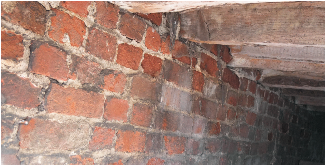
Granary under view showing west support wall of mixed bond brickwork and softwood floor joists.
