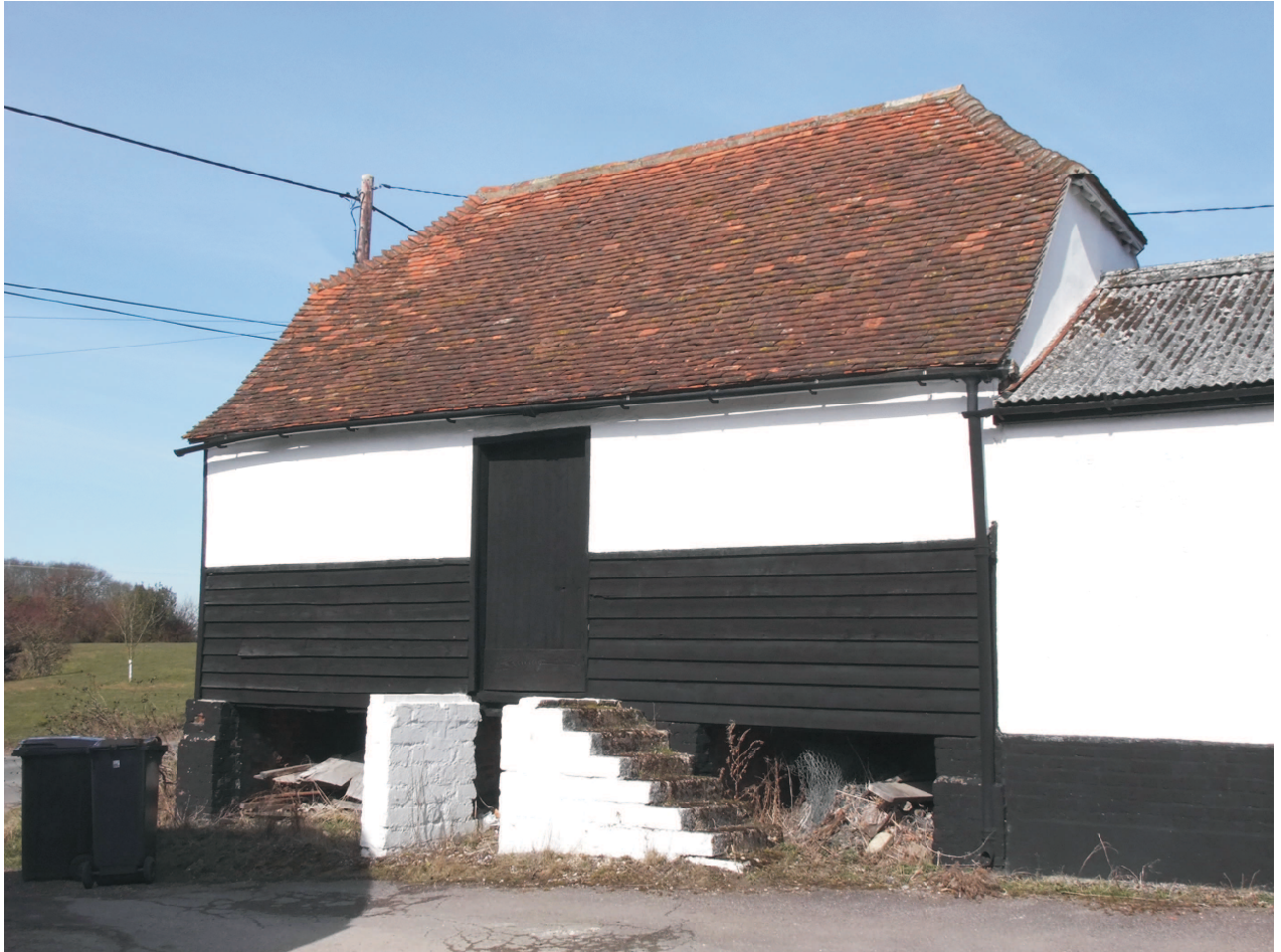
Granary south entrance side with brick formed steps to platform entrance. Pier walls return at each end and behind the steps from the intermediate walls. Weatherboarding part replaced as is plasterwork.
