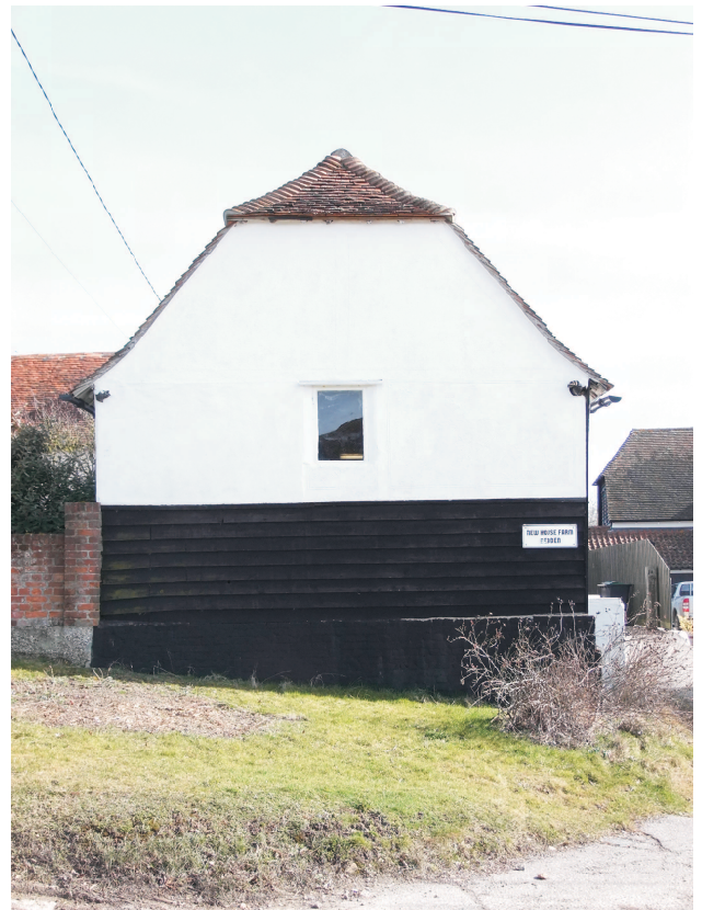
Granary west end to roadway with tarred brick plinth wall and weatherboarding and mixed age plaster above. The window is a later insertion.
