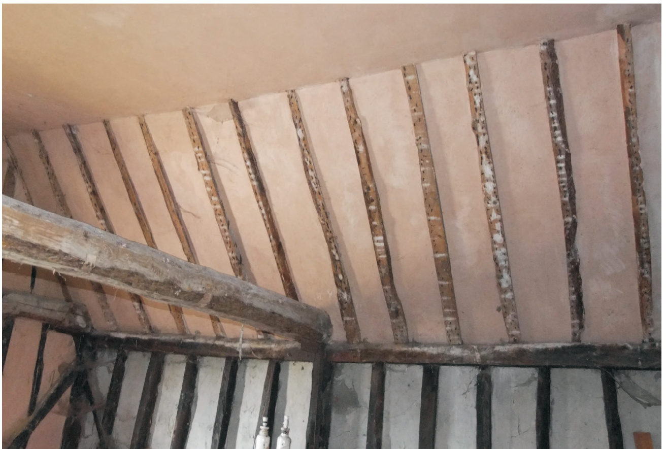
Granary view to north wall showing wall studs and wallplate. Above are rafters set evenly along the roof with no principle trusses.
