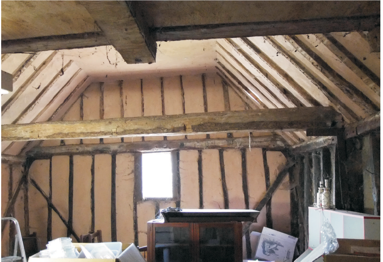
Granary long inside view to west from under inserted floor of first bay. Visible tiebeam ends have iron brackets. Primary bracing to the walls. Ceiling plastered under collar level. Inserted window in west wall.
