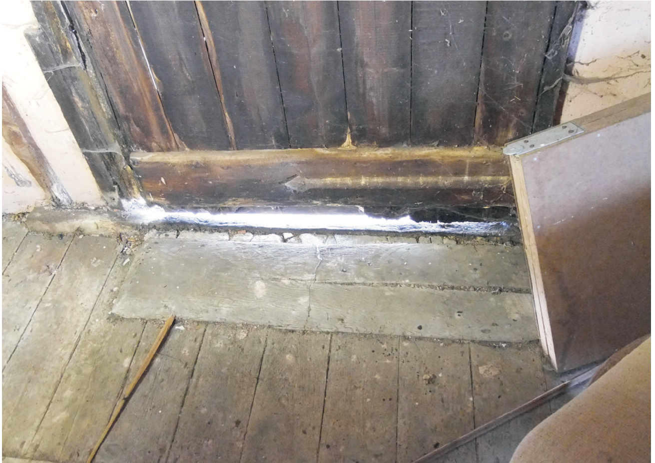
Granary south inside main door showing oak wear board fitted to floor against sill plate. 8" softwood floorboards cover floor.
