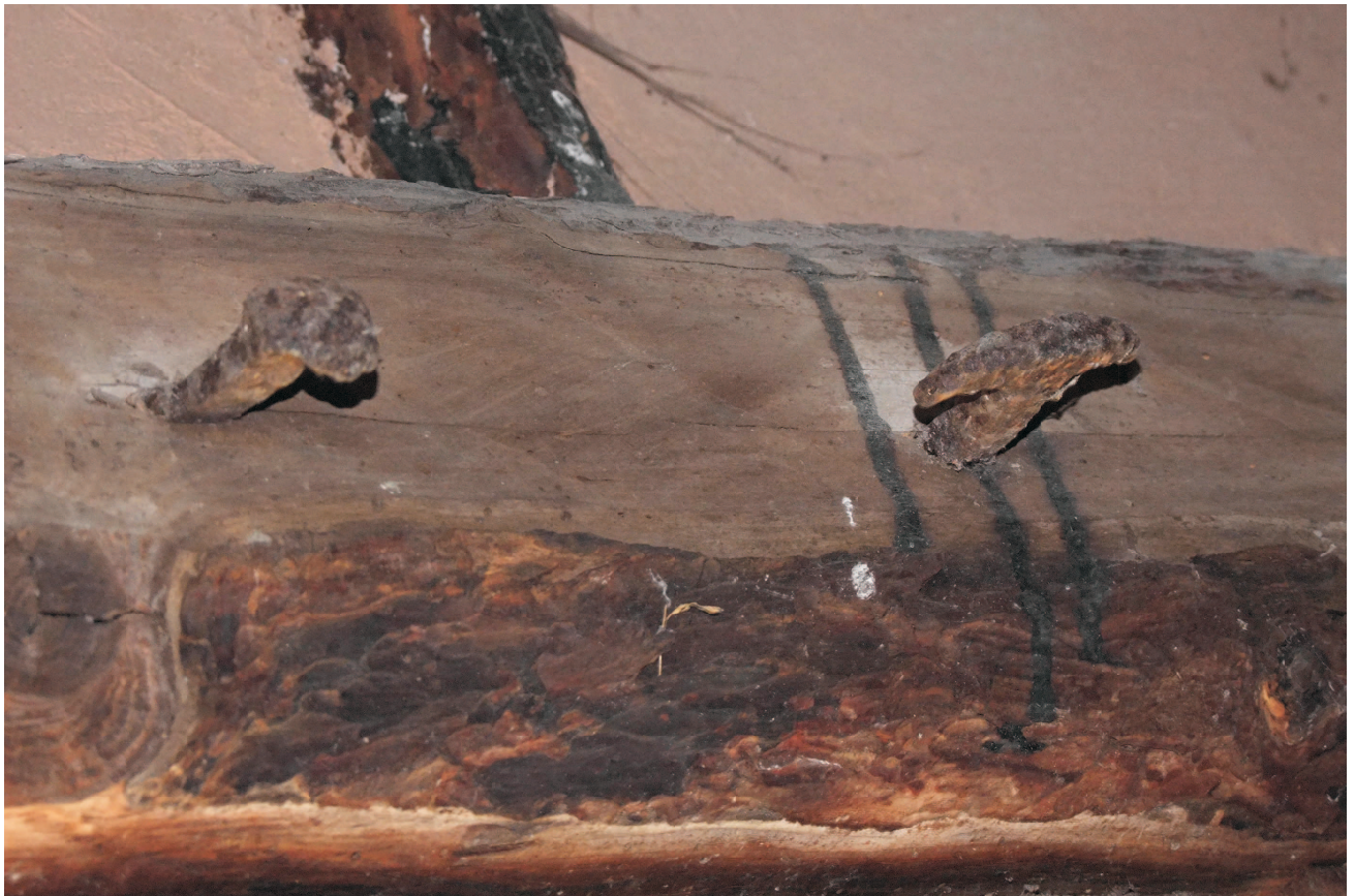
Granary tiebeam inside west end above inserted window. Iron spike and chain hook anchor fitted above window.
