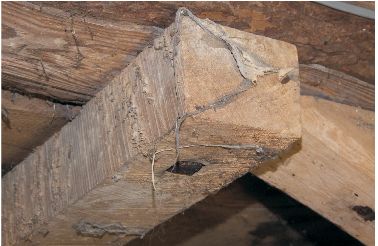
Granary detail of end of inserted joist with square head of spike let into surface. Joist and boards circular sawn.
