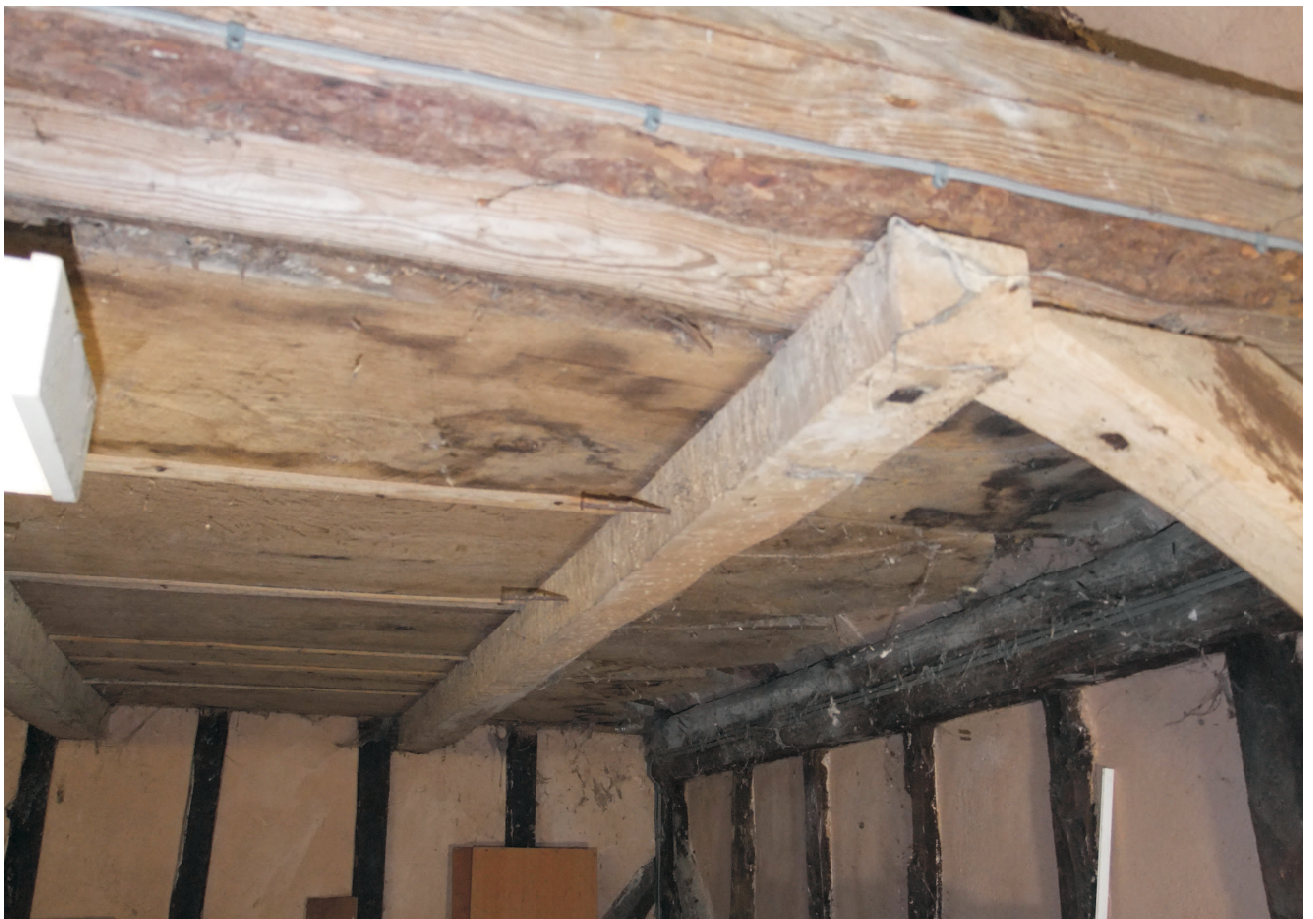
Granary view to south east corner showing inserted floor joist fitted under tiebeam.
