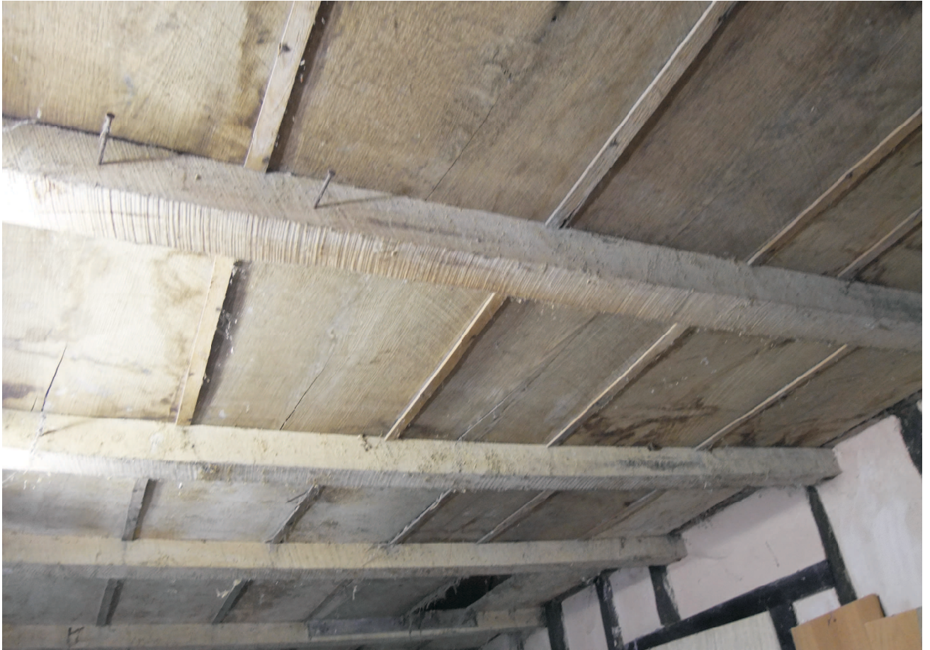
Granary inserted floor at east end showing wide short length boards with fillet strips nailed on.
