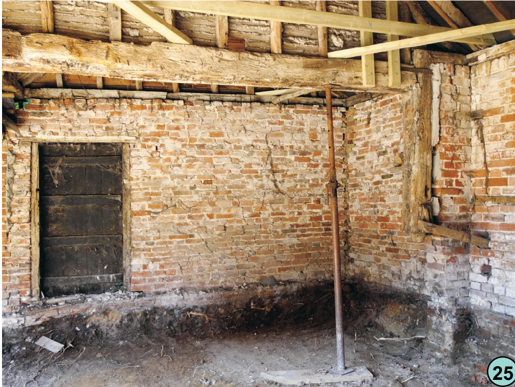
North open range view into north-west corner. Shows cut return of what was original end to this building with timber frame infill. Plastered gable to the west. Beyond this point brickwork changes and is part of the western north-south range. Door in west wall appears to be C18 so could have been moved from the end wall of the north range. This corner a closed room after C19 build.
