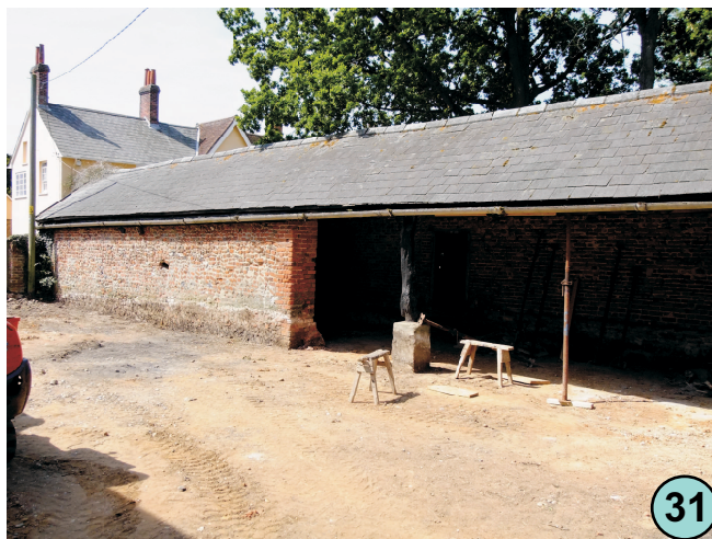
Mid C19 shelter and storage sheds to the west of the yard. Good northern quoined brick pillar to sheds but infill wall uncoursed flint and random brickwork.
