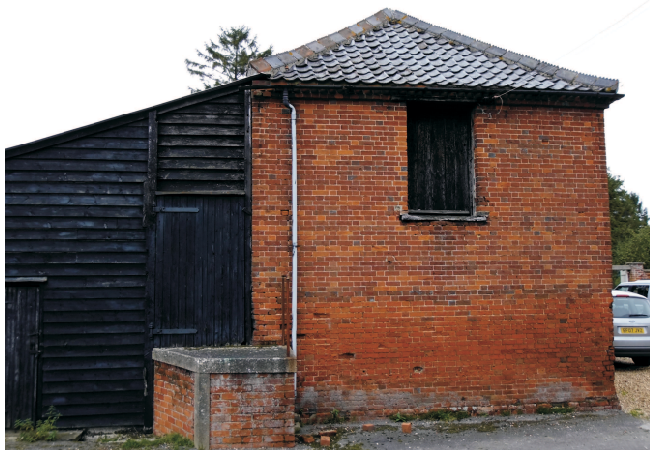
South west elevation of building with high loading door and nineteenth century lean-to addition on the rear.
