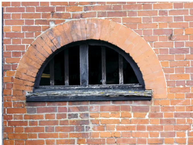
Diocletian window with rubbed brick arch, alternate bricks scored for lime putty joint.
