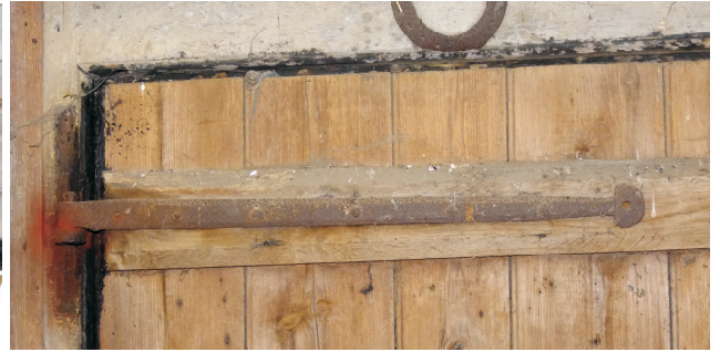
Example of one door hinge. They are clenched nailed to the door.
