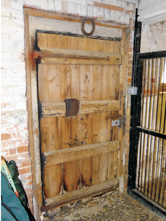
Inside of the doors, wide boards, 4 ledges & good iron work. The very long hinges do much to support the door.
