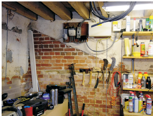
View into north corner showing scars of stall post and division structure surviving in the wall plaster. Note lacing piece in wall with long malting bricks above.
