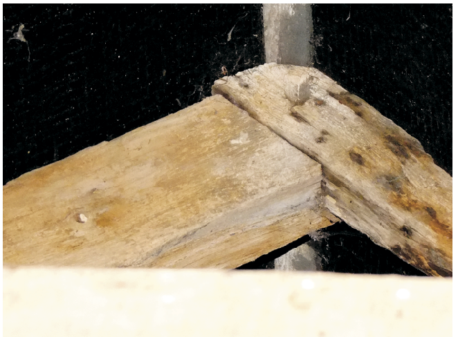
Typical apex detail for all rafter pairs. Fastened with one wooden peg. Each rafter is halved but rafter sections vary through the building.
