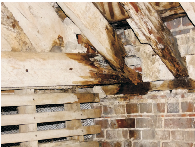
One centre bay tiebeam that has the pediment structure above. Failure of the roof detail at this point has led to much water ingress over time.
