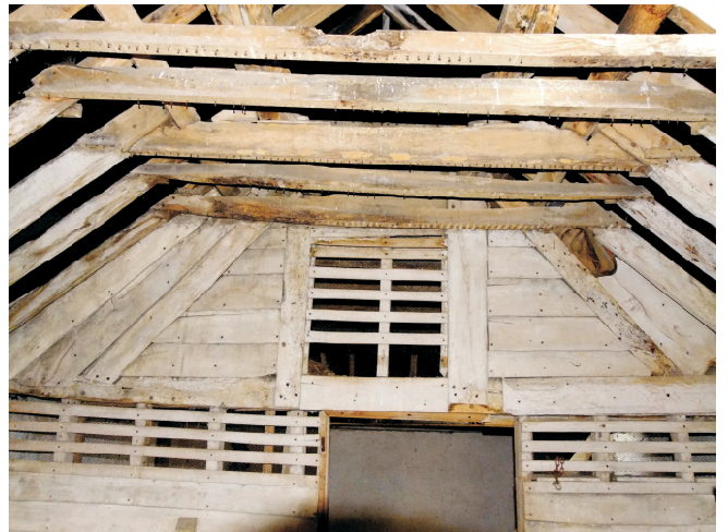
View to north east from south showing ventilated wall division to granary on line of north east side of central bay.
