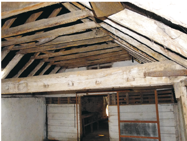
View from granary to division wall showing wide boards and vented area under tiebeam. Typical reused tiebeam in foreground with original iron ties to plate.
