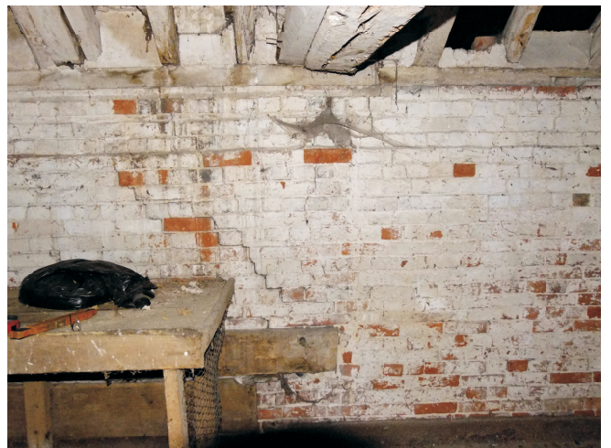
View to front showing south side of main door opening. Main opening lintol is just below table with infill boarding under to close area to floor level.
