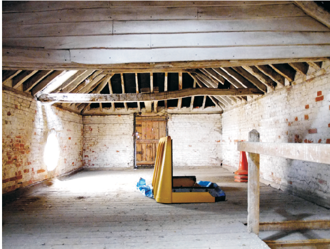
View to south west end and upper loading door. Note bay infill surviving above tiebeam to south west side of centre bay.
