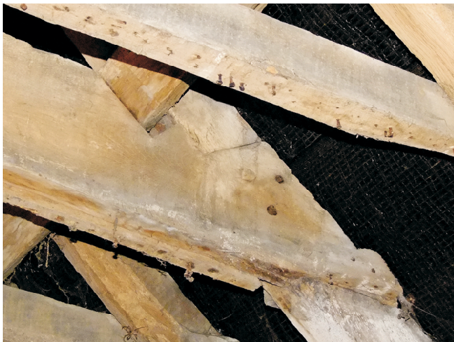
Collar detail with two wooden pegs and two nails to each end. Purlin clasped by rafter and collar.
