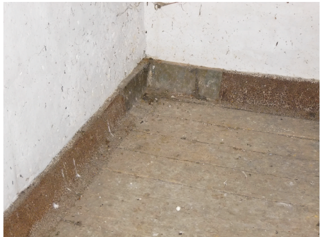
Granary floor area showing plastered walls and wooden floor junction sealed with sheet iron edging.
