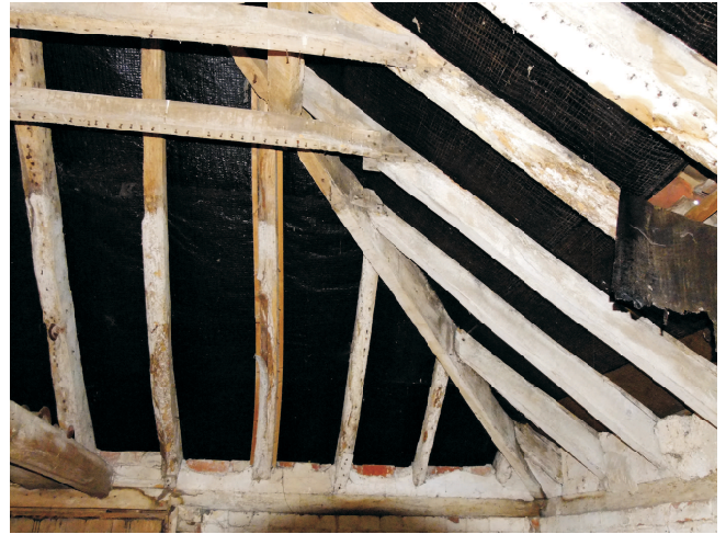
Typical hip construction. Lime wash stain shows original plaster level to under collars.
