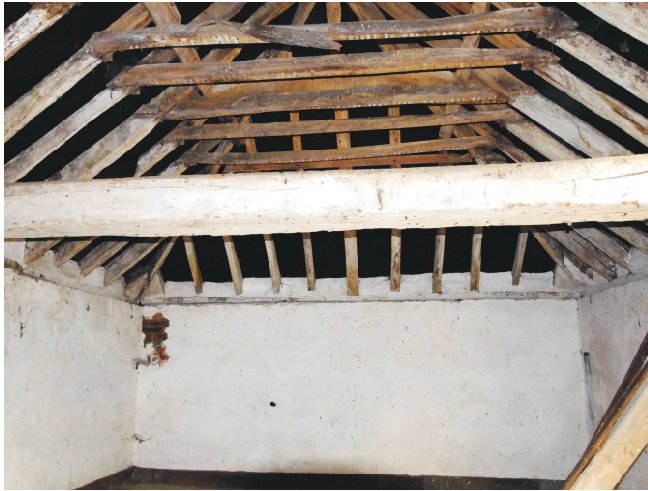
First floor view to north east showing granary end with fully plastered walls. Ceiling joists nailed to each rafter pair for plaster with undersides in line with lower face of collars.
