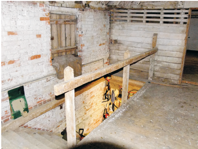
Inserted staircase and floor to central bay with handrail. 'Pitching' door is in the centre of this area.
