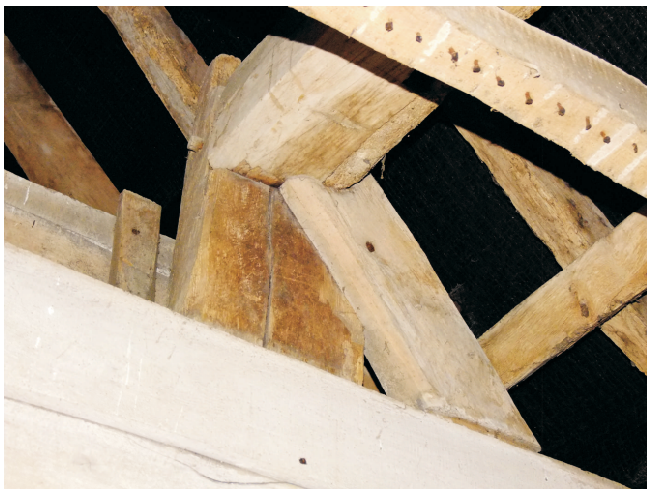
Detail of top construction with main beams mortised and tenoned into vertical posts and braces keyed under apparently only nailed.
