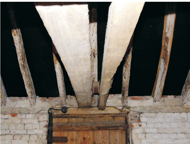
Beams at south west end to upper loading door supported back to first tiebeam
