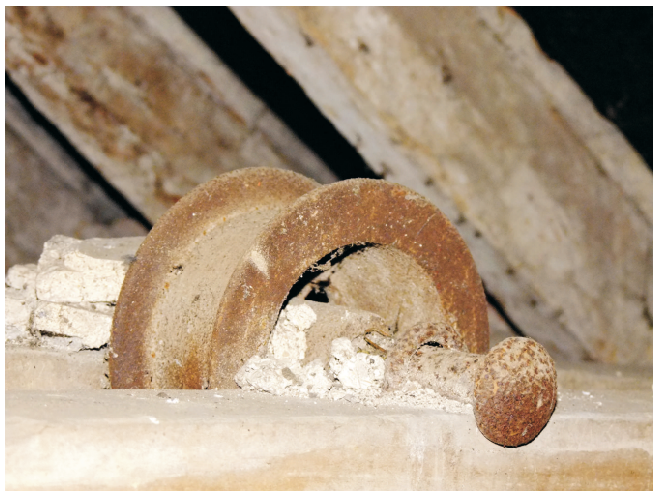
Detail of pulley mounting set towards opening and on top of beams.
