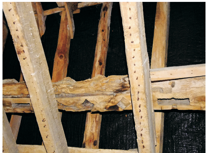
Detail of one reused beam showing mortises for window mullions and channel for sliding shutter with stud mortises to either side.
