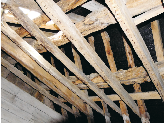
Two heavy reused beams in central bay set over collar level. Suggested use is for a hoist.
