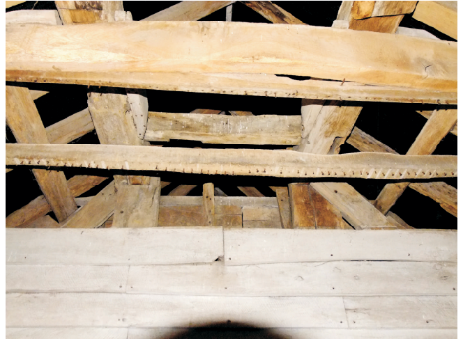
End support system for beams. Vertical post from tiebeam with bracing from top to tiebeam and tie piece between the beams.
