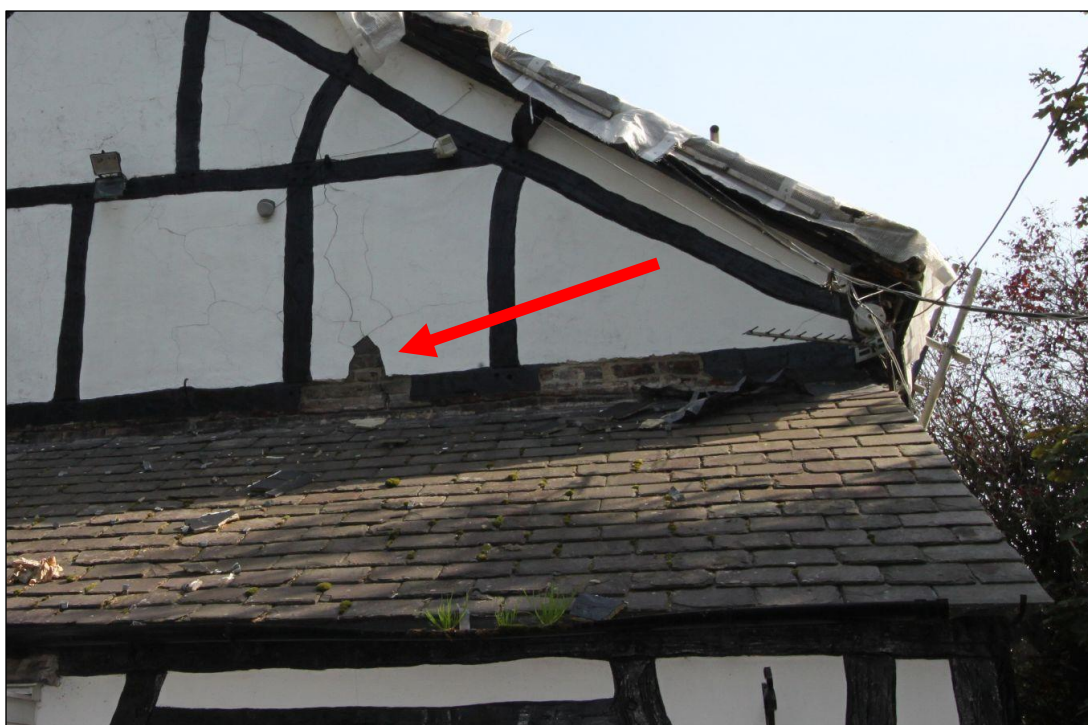
Plate 21: Handmade brick exposed behind applied Mock Tudor timber frame, on western gable
