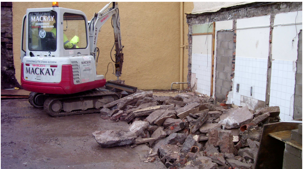
Plate 13: View to the south-west showing machine excavation of toilet extension, and concrete 1029 , drains 1031 and rubble levelling material 1030
