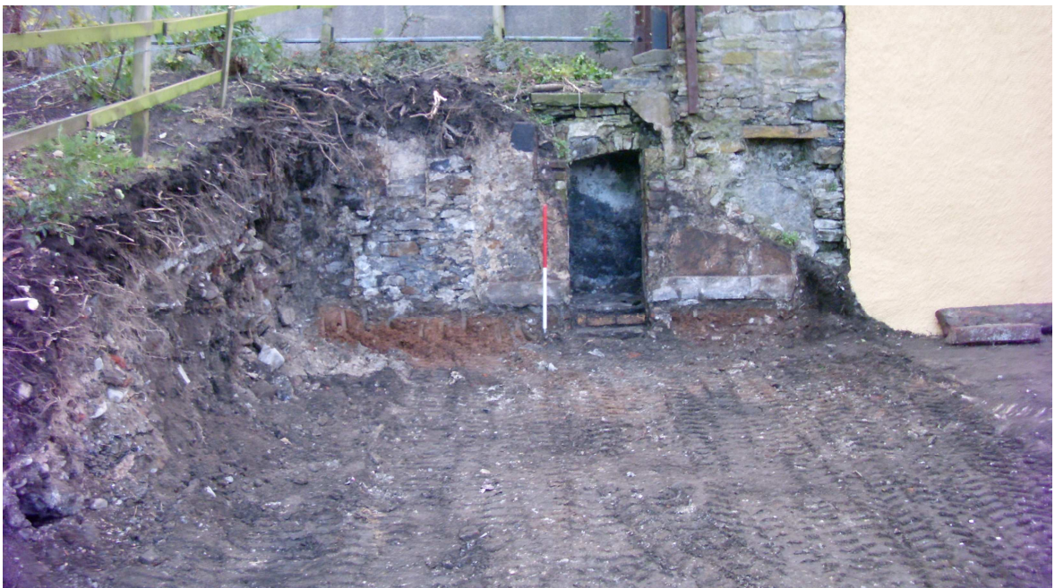
Plate 7: View to the south-east of landscaped bank 1035 , tenement wall 1034 , and coal cellar 1033 , exposed by ground reduction
