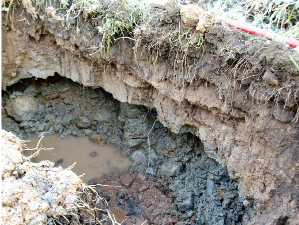
Plate 1: South-west facing section of TP201, Storage pond site, showing unstable ground conditions
