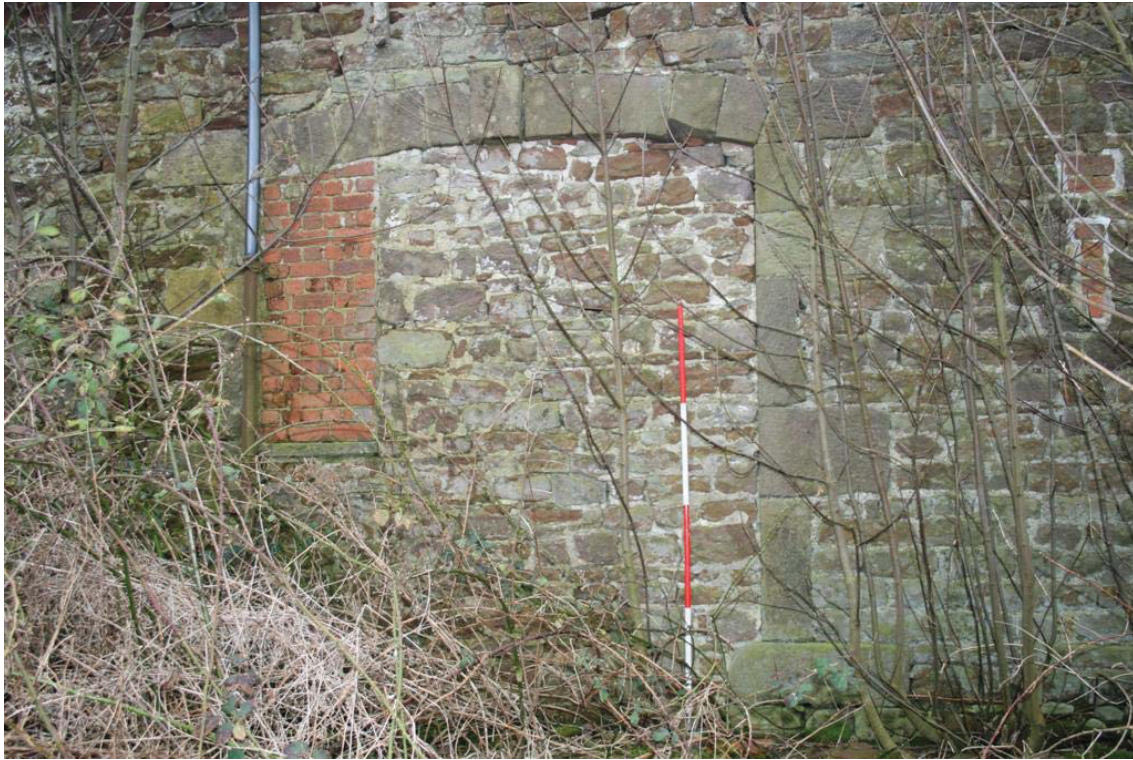
Plate 5: Blocked door and window on the west facing elevation of Barn A
