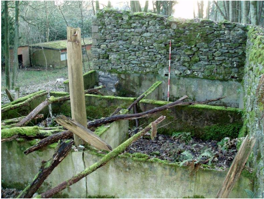
Plate 45: Interior of the derelict structure, Building 5
