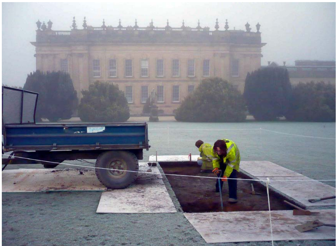
Plate 4: Trench 2 being excavated on one of the many frosty mornings at Chatsworth, the east front of the house can be seen in the background
