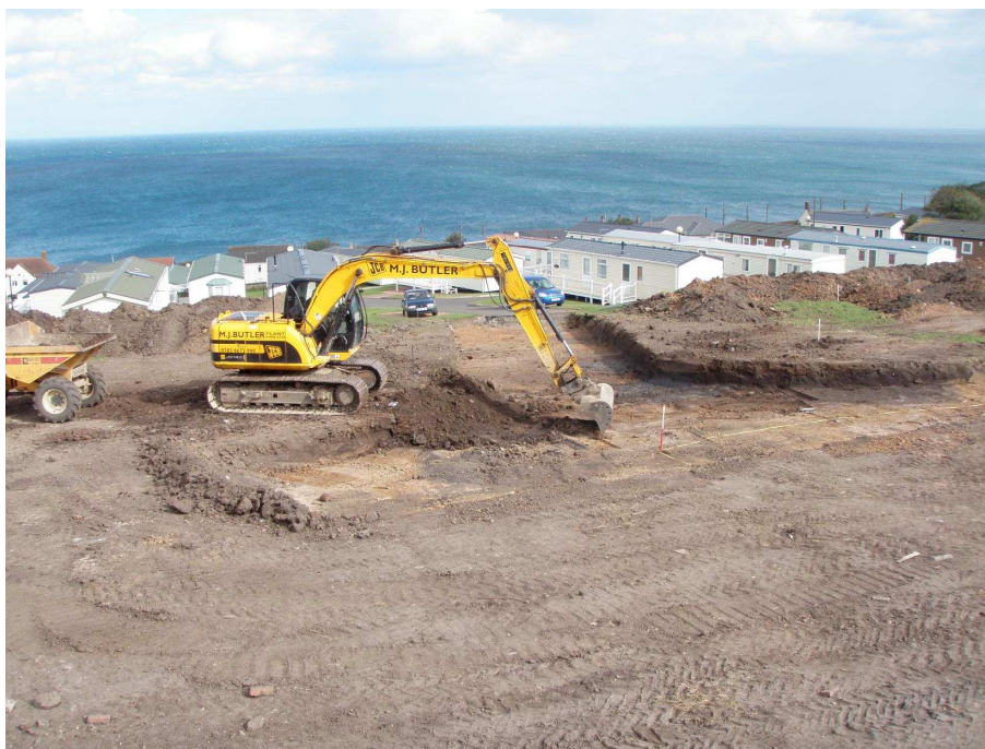
Plate 1: Excavation of haul roads at the eastern end of the site. Pits 26 and 27 can be seen to the immediate right of the machine's bucket
