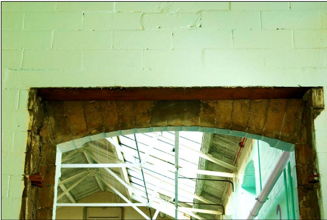
Plate 64: Segmental arch of the doorway from Room 100 to Room 60 in the Science Building
