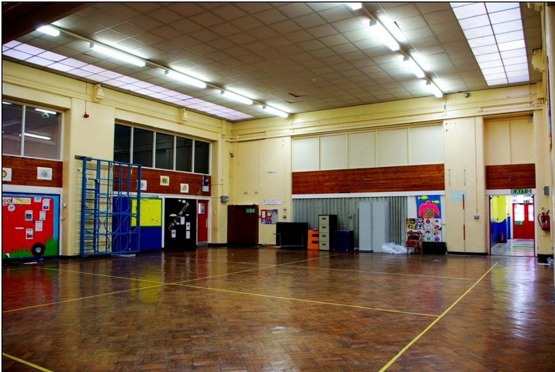
Plate 36: View of the main hall in the Junior School prior to stripping (facing north-east)
