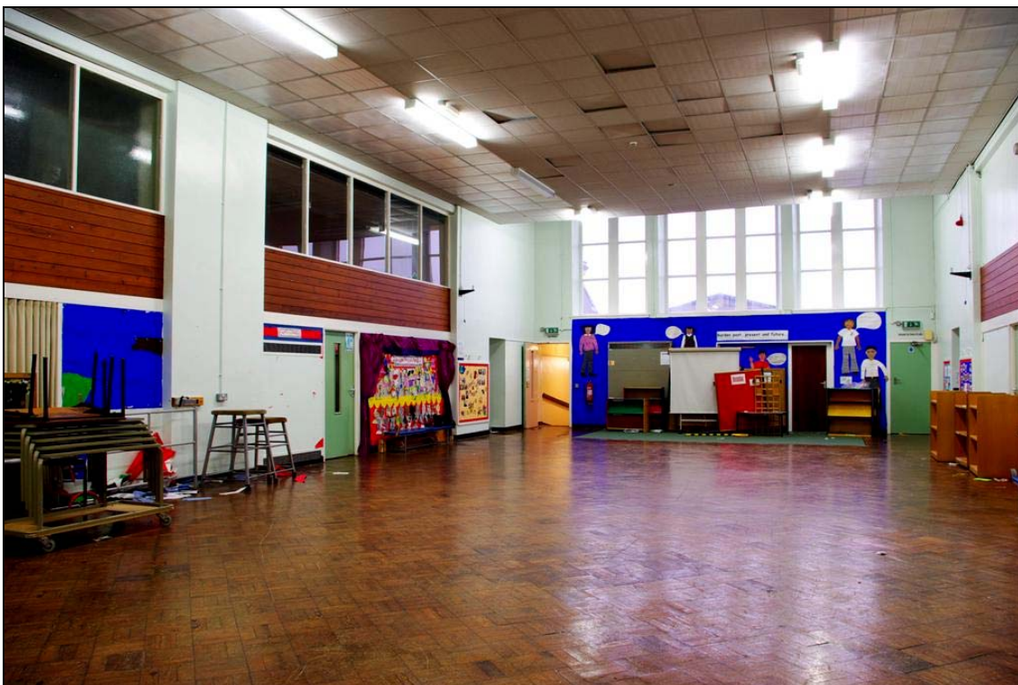
Plate 55: General view of the main hall (Room 29) in the Infants School (facing north) prior to stripping
