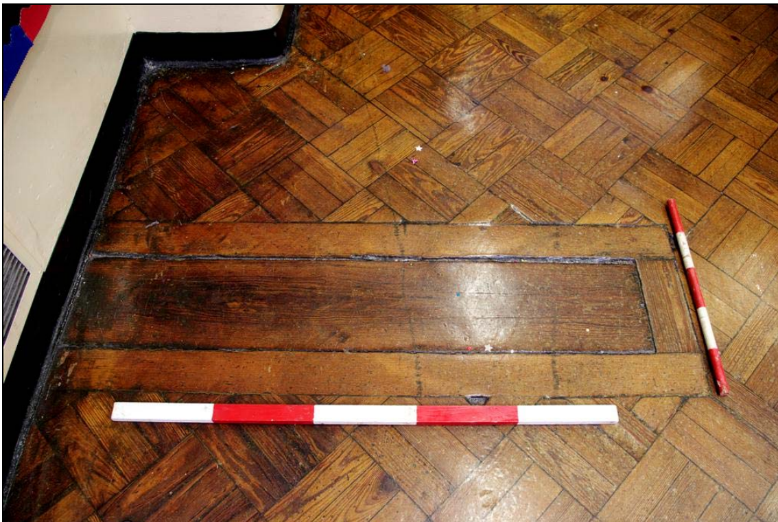
Plate 37: Access to heating pipes in the main hall
