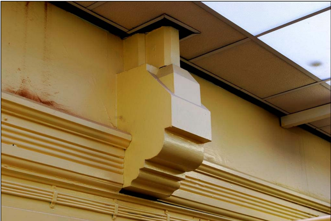
Plate 43: Corbel which supports the truss in the main hall of the Junior School
