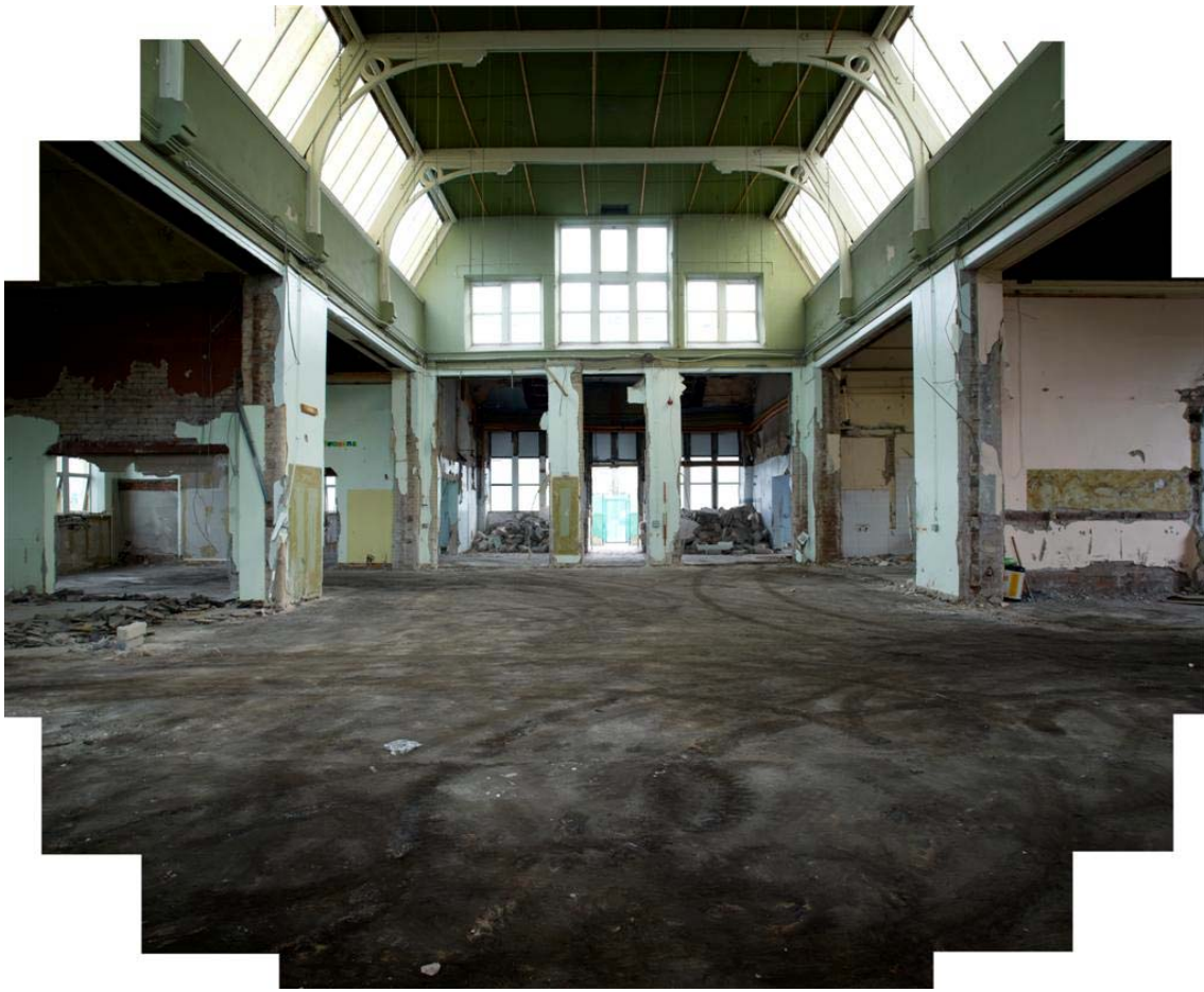
Plate 56: Composite view of the main hall in the Infants School (Room 29) facing south
