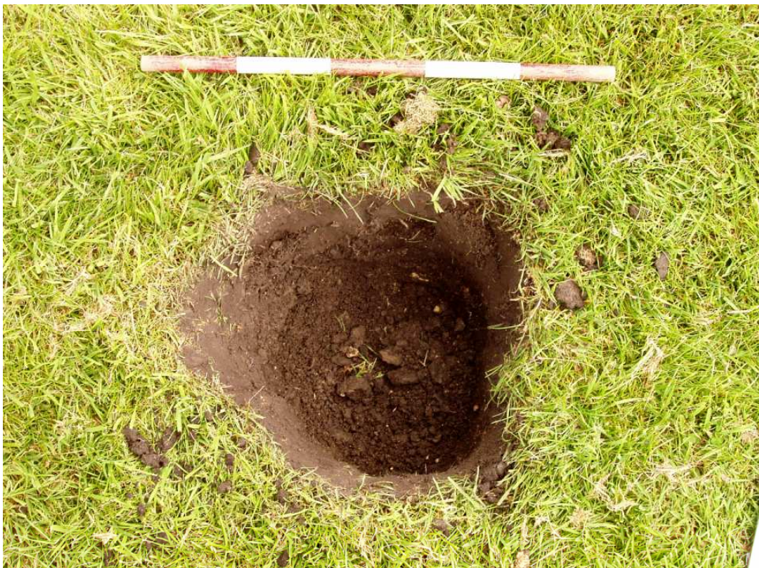
Plate 6: A post hole excavated for the 'Abbey Refectory' interpretation sign (location 5) at Sawley Abbey facing east
