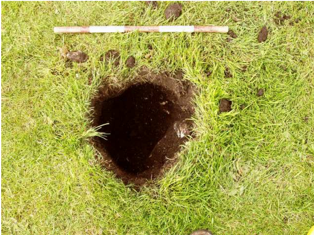
Plate 4: A post hole excavated for the 'Welcome to Sawley Abbey' interpretation sign (location 3), facing north-west
