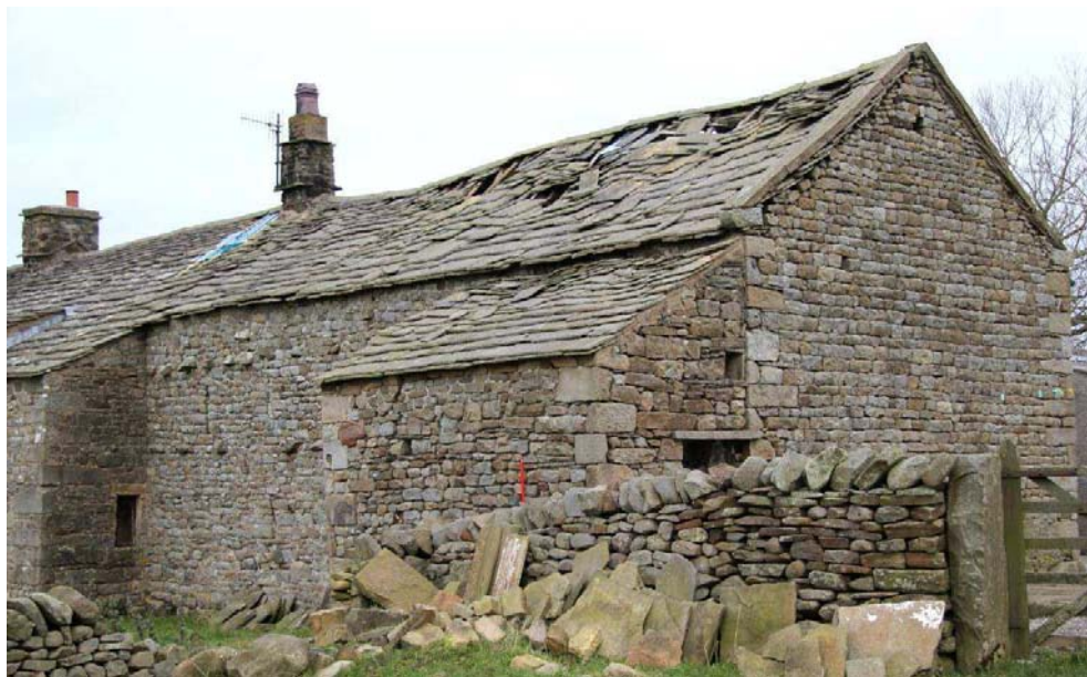
Plate 5: Oblique view of the east side of the barn and the lean-to
